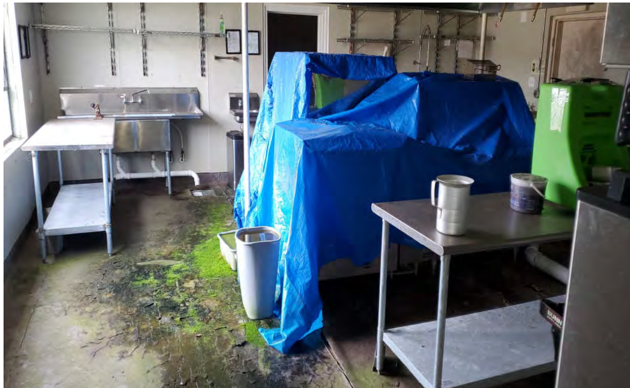
Photograph 13 - Typical Moisture Damage & Mold Growth in Cafeteria from Damaged Roof.
