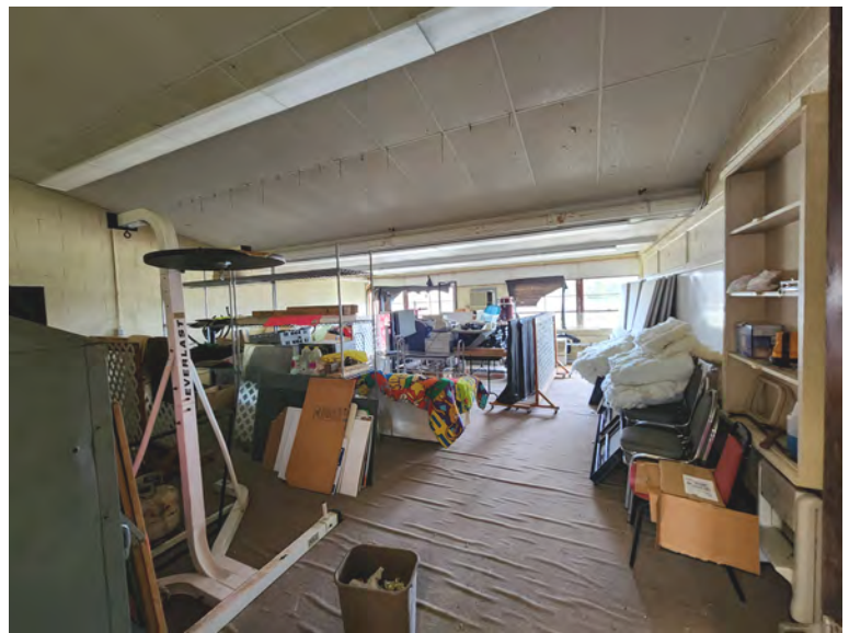
Classroom with evidence of moisture throughout (wrinkled carpet, smell, visible mold, etc.)
