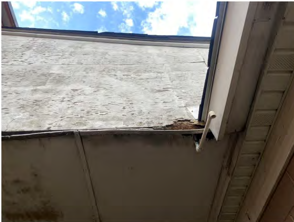
Photograph 12 – Damaged Soffit/Fascia Area at Rear of Gym/Classroom Connector
