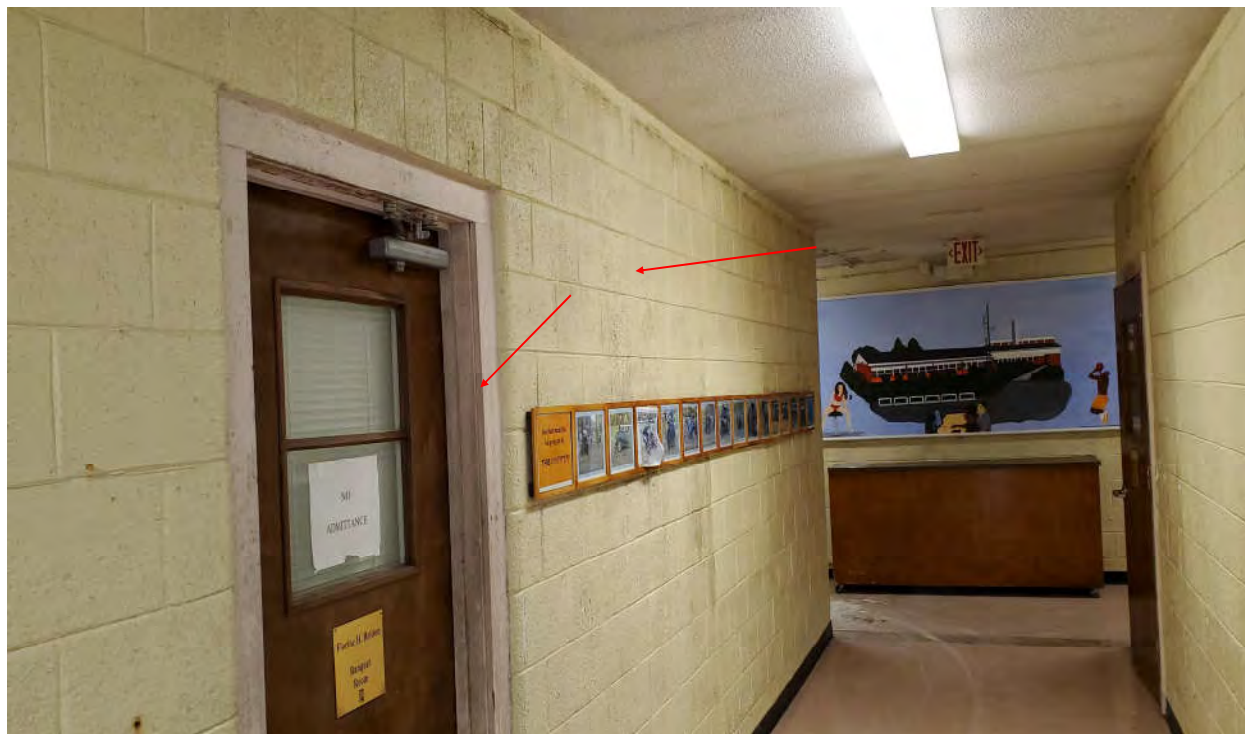
Photograph 9 - Typical Mold Growth on Walls, Door Components, & Other Surfaces Located Throughout the Main Building.
