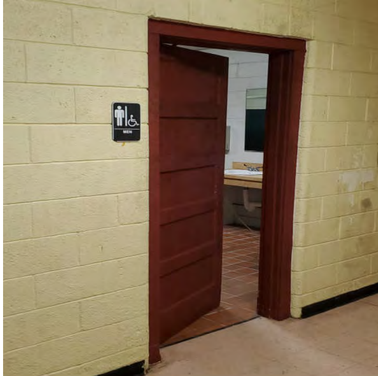
Photograph 7 - Typical Lead-Based Paint on Red Doors and Dooring Casings in Restrooms of Main Building.
