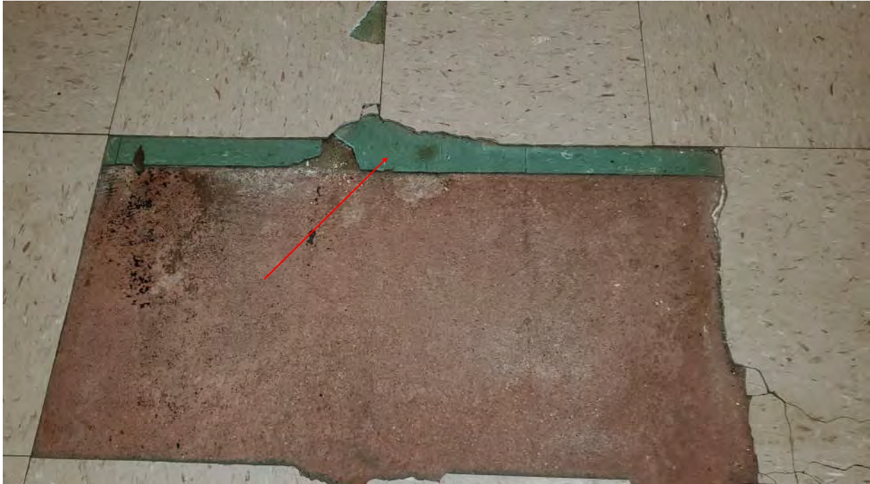
Photograph 3 - Homogeneous Area A-06 - Typical Asbestos-Containing 9" x 9" Floor Tile & Black Mastic (Green & Brown Colors) Located as Underlayer Throughout Main Building Classrooms, Corridors, & Office Area Under Carpet or Non-ACM Floor Tile or Linoleum
