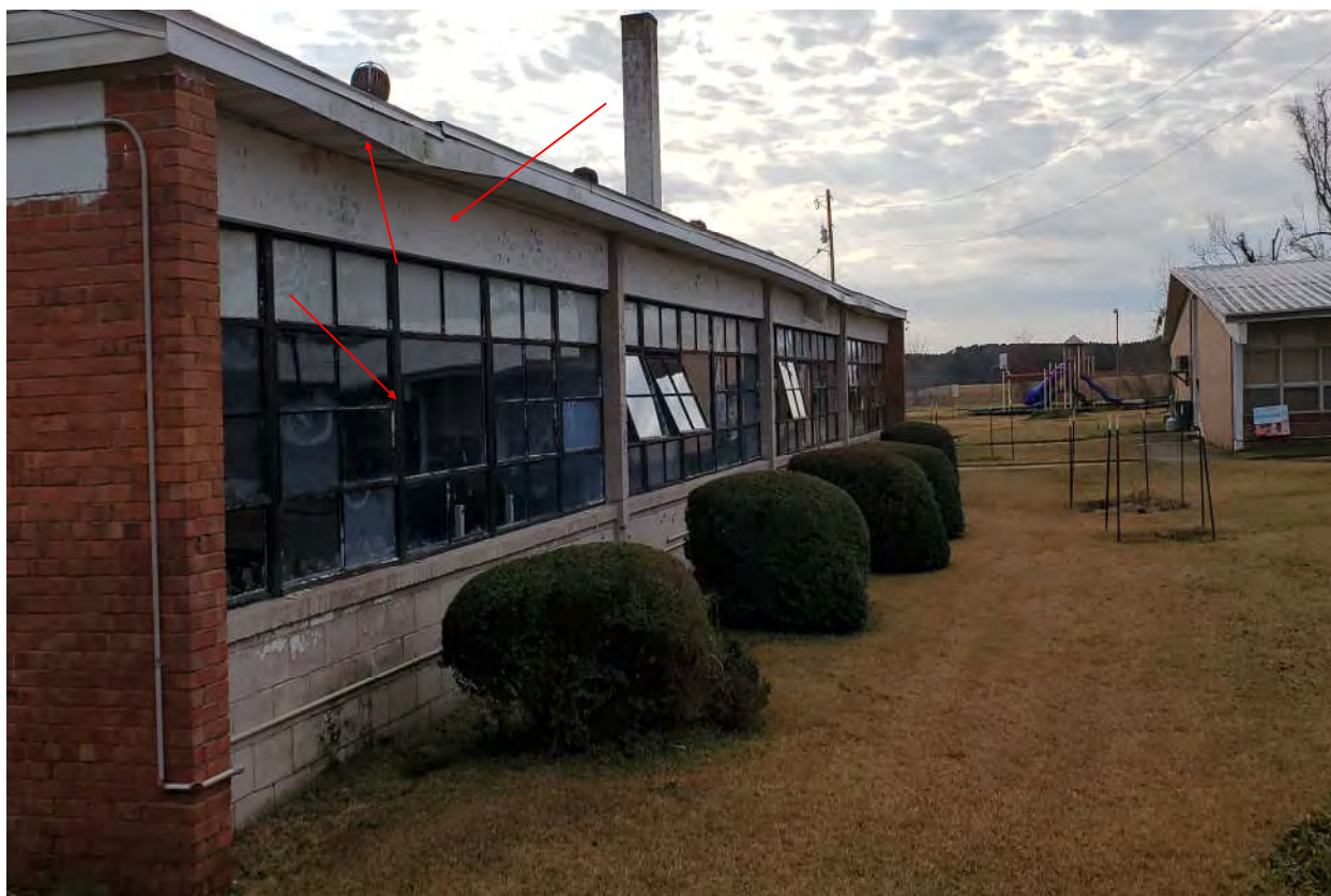
Photograph 6 - Typical Lead-Based Paint Throughout Interior and Exterior Metal Window Components (Sashes & Casings), Concrete Window Headers, & Wooden Eaves of Main Building.
