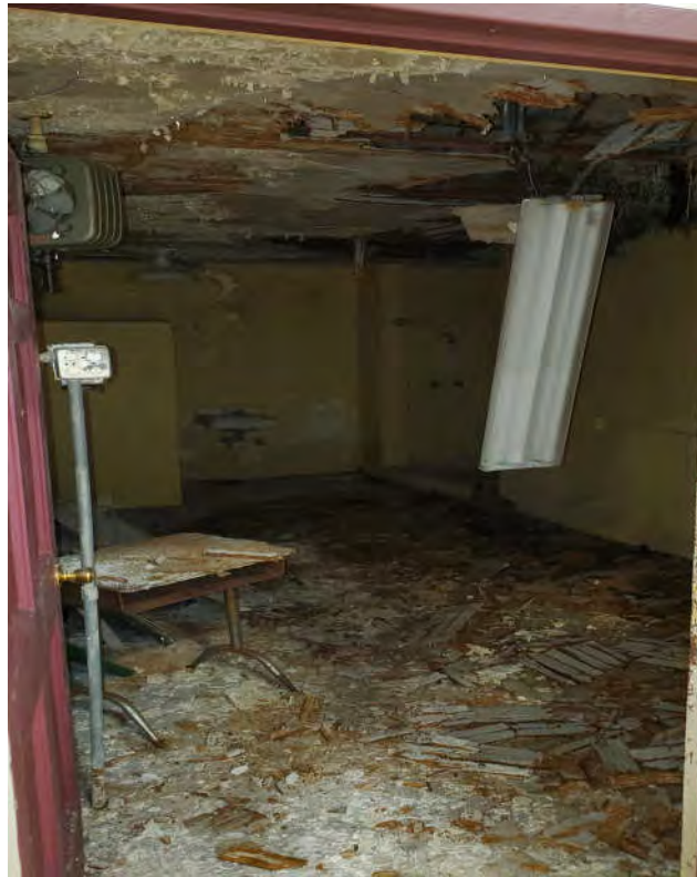
Photograph 16 - Typical Moisture Damage & Mold Growth on Walls, Door Components, & Other Surfaces in the Gym Locker Rooms from Damaged Roof.
