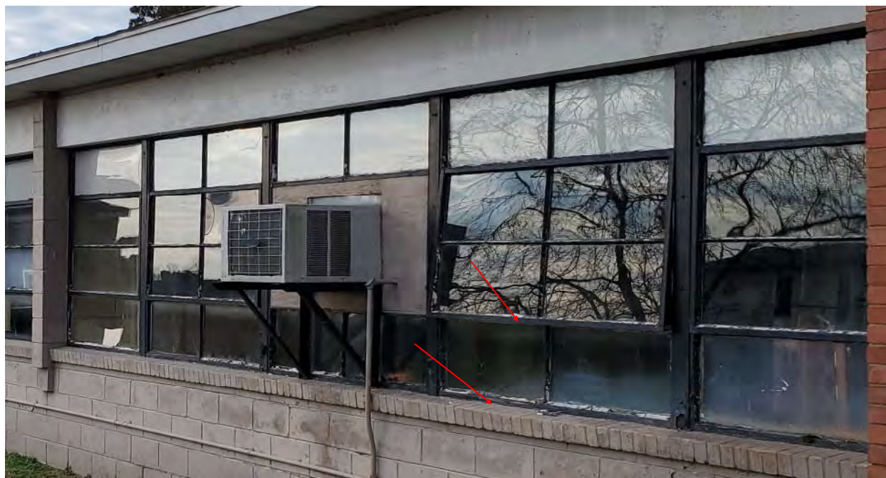
Photograph 1 - Homogeneous Areas A-01 & A-22—Typical Asbestos-Containing Exterior Window Glazing and Window Frame Caulking Located Throughout Main Building Window Units. (57 Window Units)
