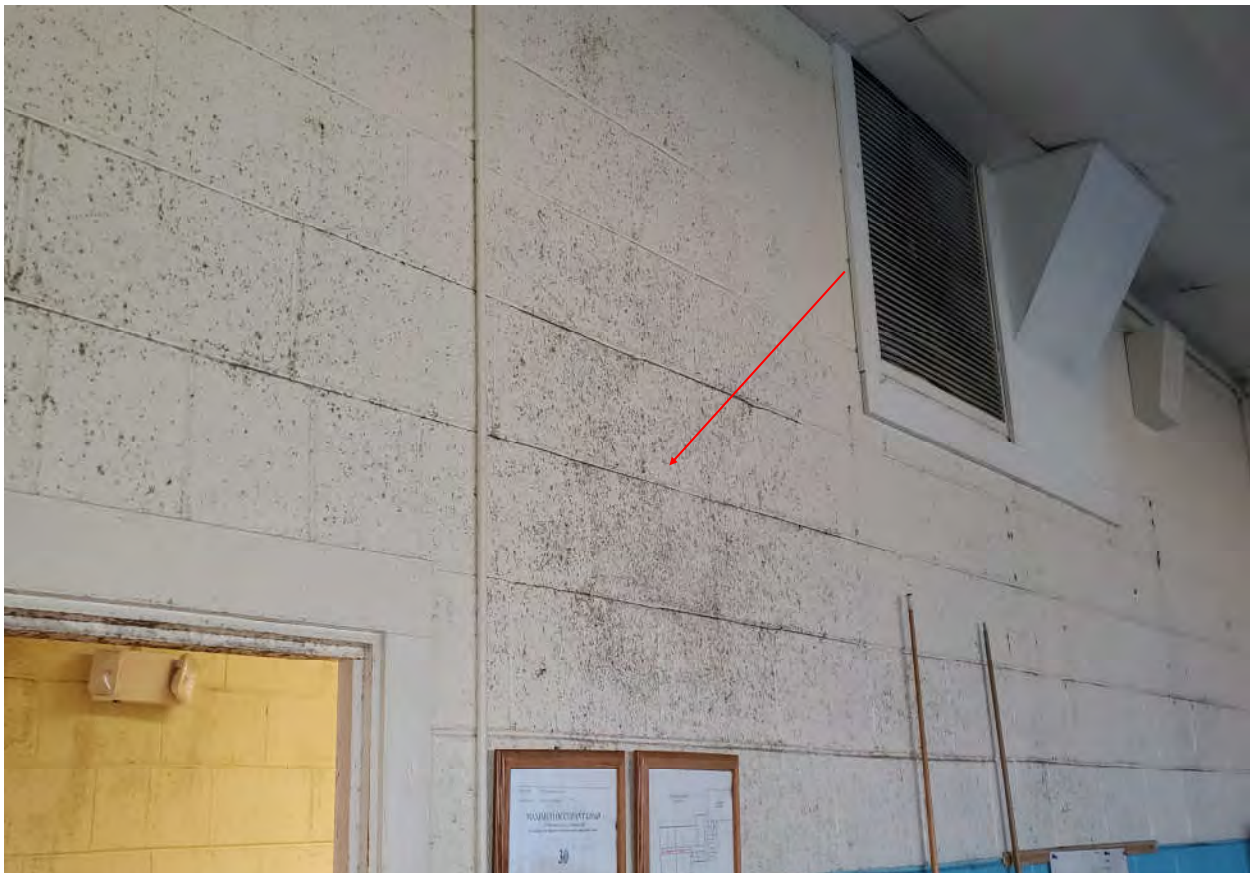
Photograph 12 - Typical Mold Growth on Walls, Door Components, & Other Surfaces Located Throughout the Main Building.
