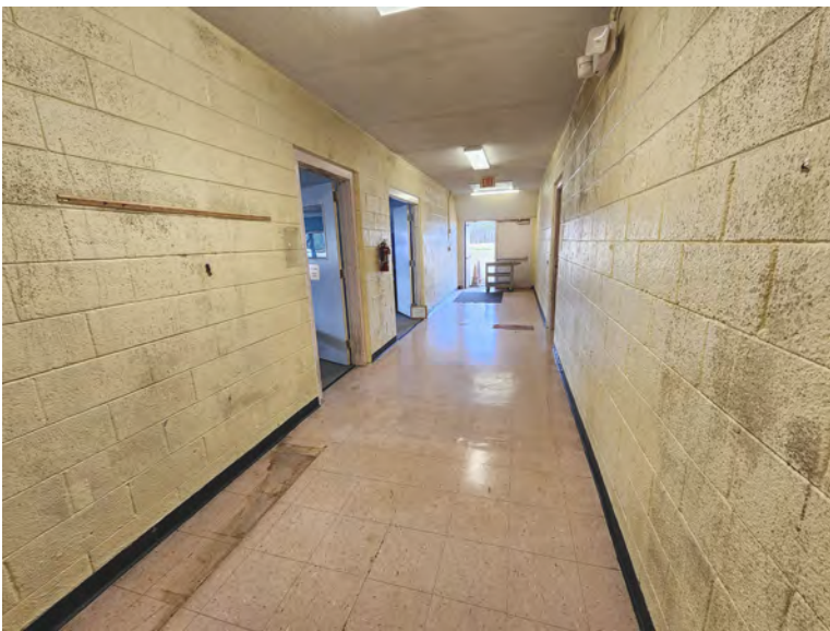
Classroom hallway with visible mold on walls.
