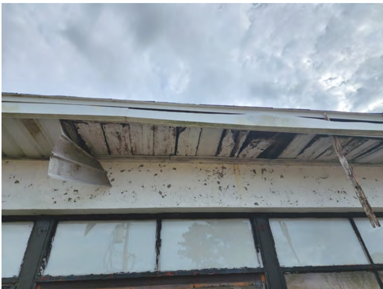
deteriorating soffit condition.
