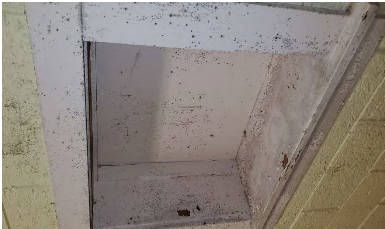
Photograph 11 - Typical Mold Growth on Walls, Door Components, & Other Surfaces Located Throughout the Main Building.
