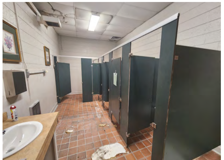
Existing Women's Restroom - Minor ADA compliance concerns.
