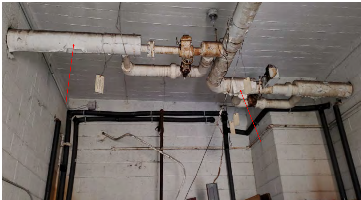
Photograph 5 - Homogeneous Area A-23 - Asbestos-Containing “Air-Cell” Straight Run Pipe Insulation Located Overhead in the Mechanical Room. (10 LF)
