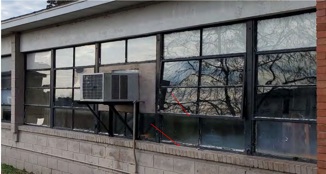
Photograph 1 - Homogeneous Areas A-01 & A-22—Typical Asbestos-Containing Exterior Window Glazing and Window Frame Caulking Located Throughout Main Building Window Units. (57 Window Units)
