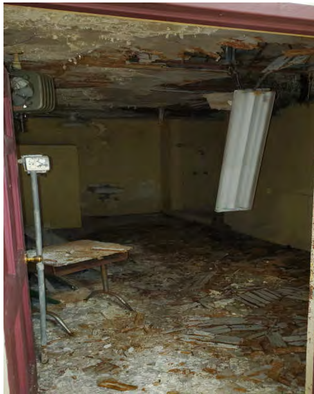
Photograph 16 - Typical Moisture Damage & Mold Growth on Walls, Door Components, & Other Surfaces in the Gym Locker Rooms from Damaged Roof.
