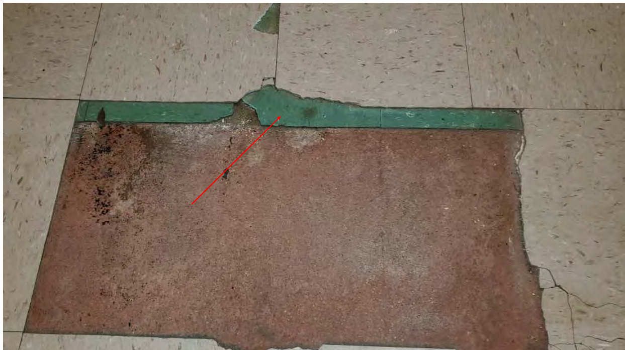
Photograph 3 - Homogeneous Area A-06 - Typical Asbestos-Containing 9" x 9" Floor Tile & Black Mastic (Green & Brown Colors) Located as Underlayer Throughout Main Building Classrooms, Corridors, & Office Area Under Carpet or Non-ACM Floor Tile or Linoleum
