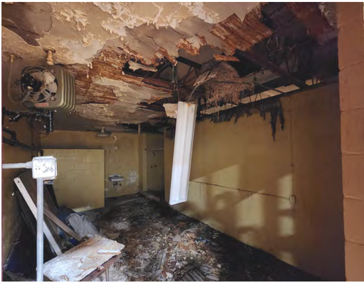
Water damage to locker rooms.
