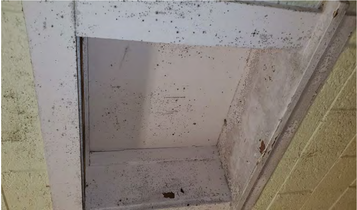
Photograph 11 - Typical Mold Growth on Walls, Door Components, & Other Surfaces Located Throughout the Main Building.
