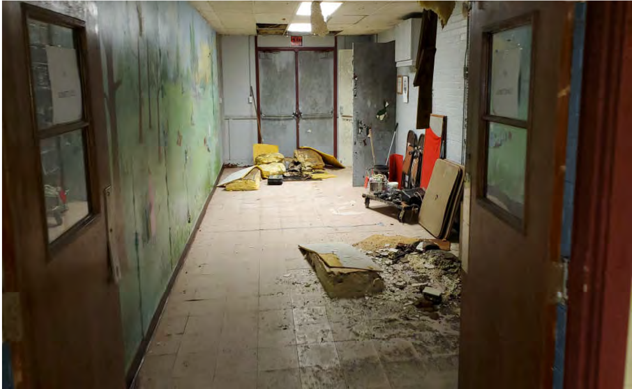
Photograph 15 - Typical Water Damage & Mold Growth in Gym Corridor from Damaged Roof.
