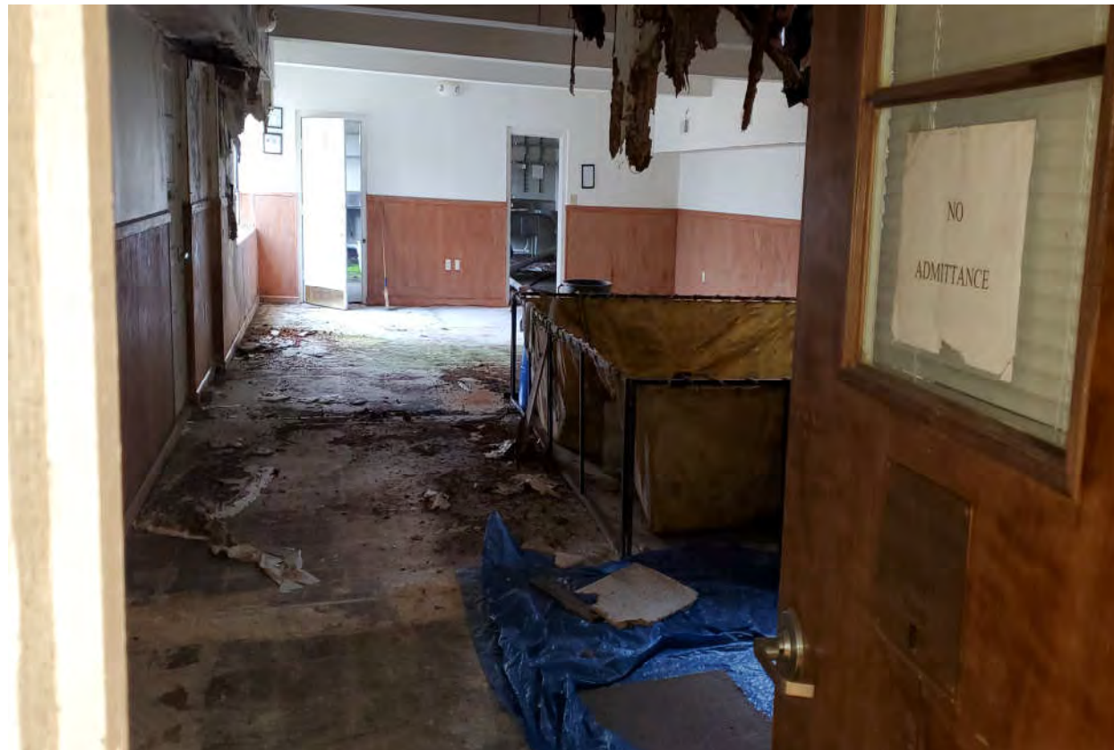
Photograph 14 - Typical Moisture Damage & Mold Growth on Walls, Door Components, & Other Surfaces in the Cafeteria from Damaged Roof.
