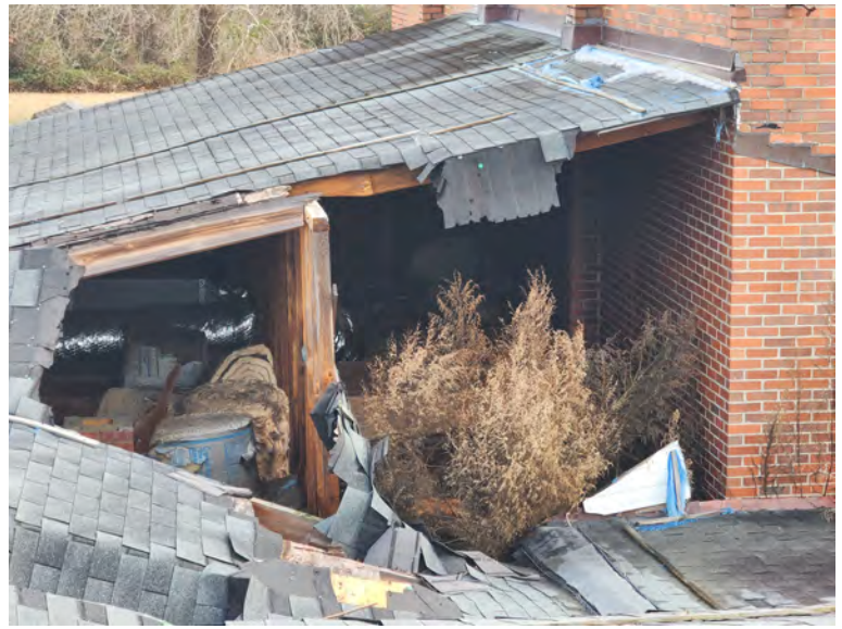
Roof collapse view from the roof.
