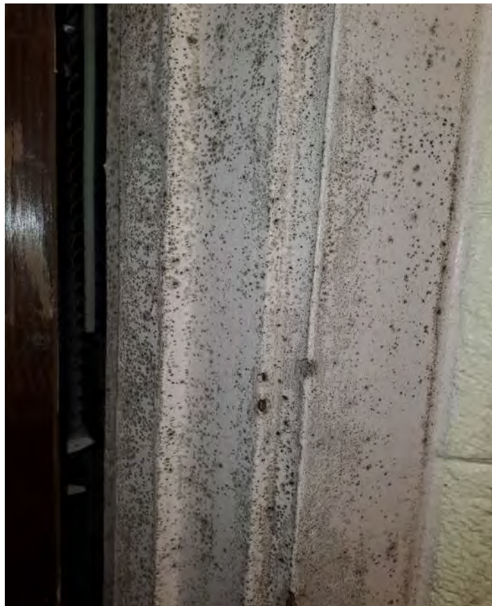
Photograph 10 - Typical Mold Growth on Walls, Door Components, & Other Surfaces Located Throughout the Main Building.
