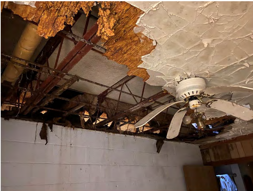
Photograph 16 – Damaged Ceiling and Rusted Bar Joists at Gym Locker Room Area
