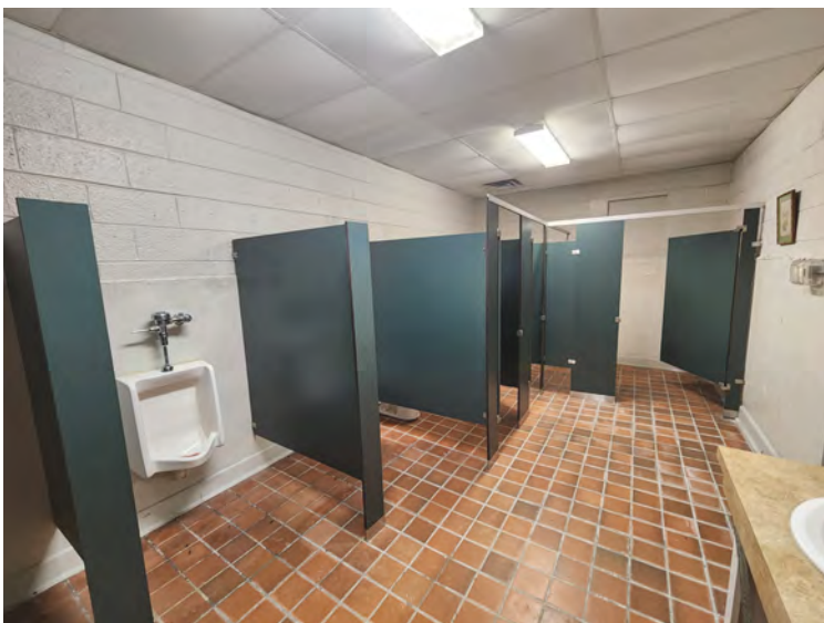
Existing Men's Restroom - Minor ADA compliance concerns.
