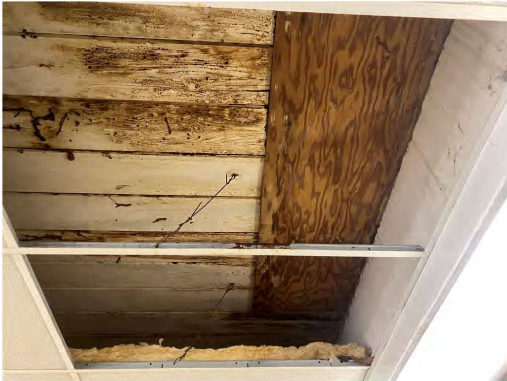
Photograph 14 – Roof Sheathing Damage/Patch Near Front/Center of Classroom Bldg
