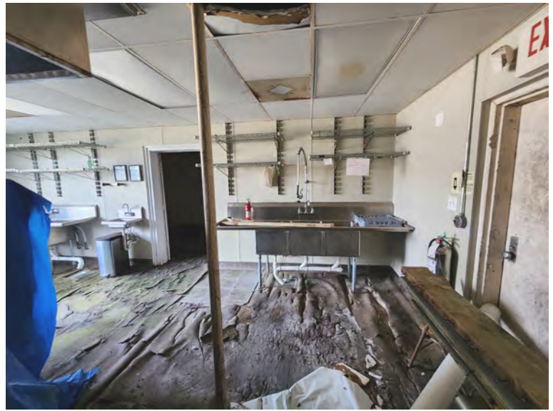
Water damage to commercial kitchen.
