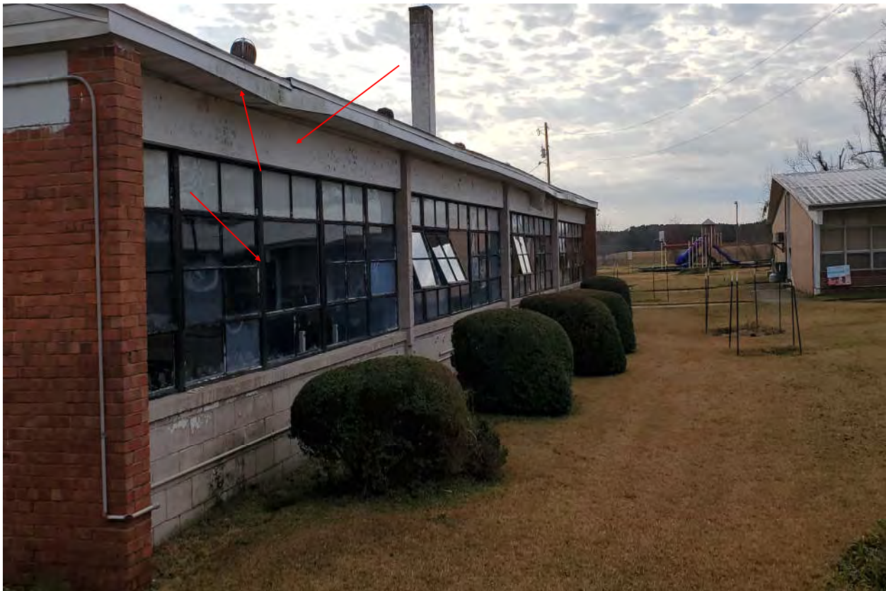
Photograph 6 - Typical Lead-Based Paint Throughout Interior and Exterior Metal Window Components (Sashes & Casings), Concrete Window Headers, & Wooden Eaves of Main Building.
