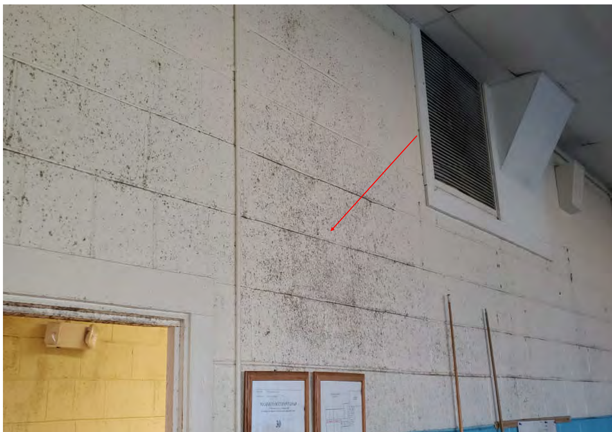
Photograph 12 - Typical Mold Growth on Walls, Door Components, & Other Surfaces Located Throughout the Main Building.
