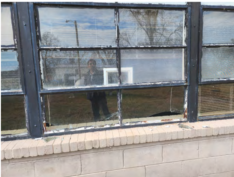
Broken window glass and rotted sashes.
