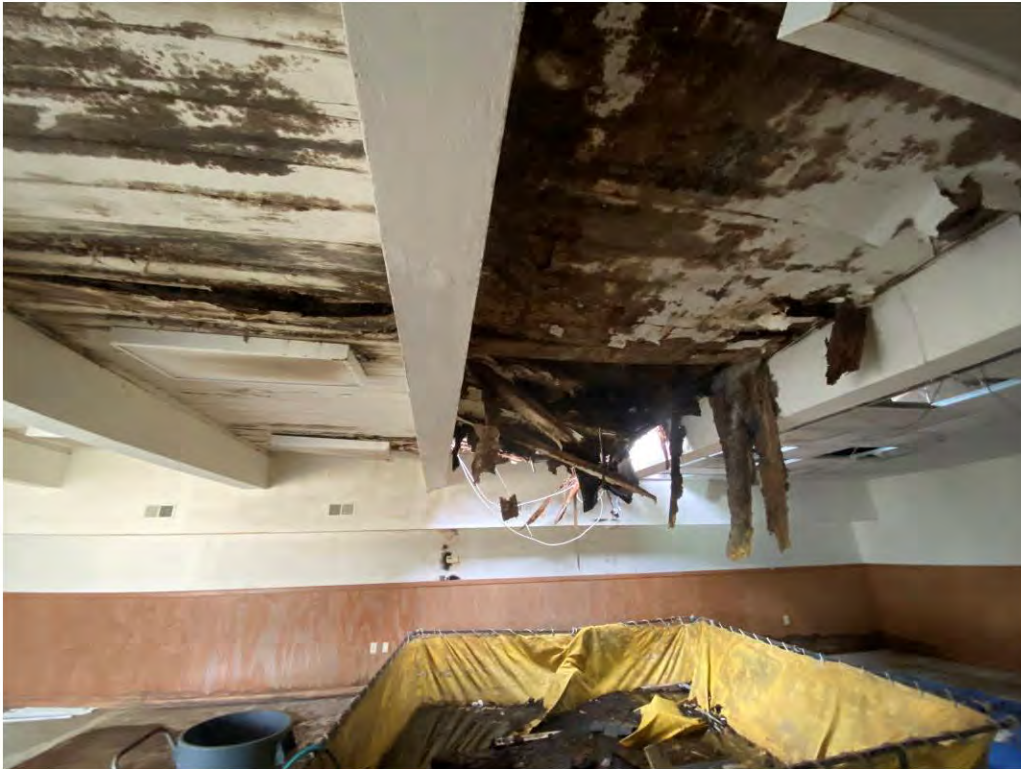
Photograph 15 – Damaged Original Roof Sheathing at Right End of Classroom Building
