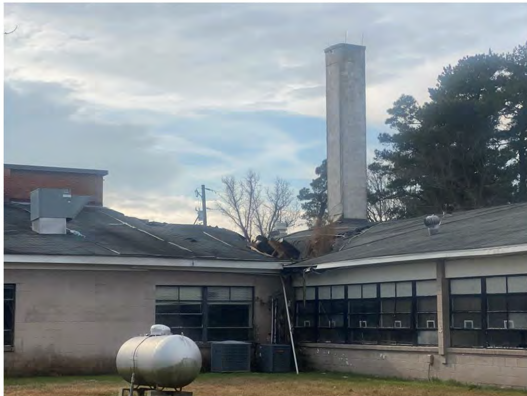
Photograph 10 – Collapsed Roof Area at Right End of Classroom Building
