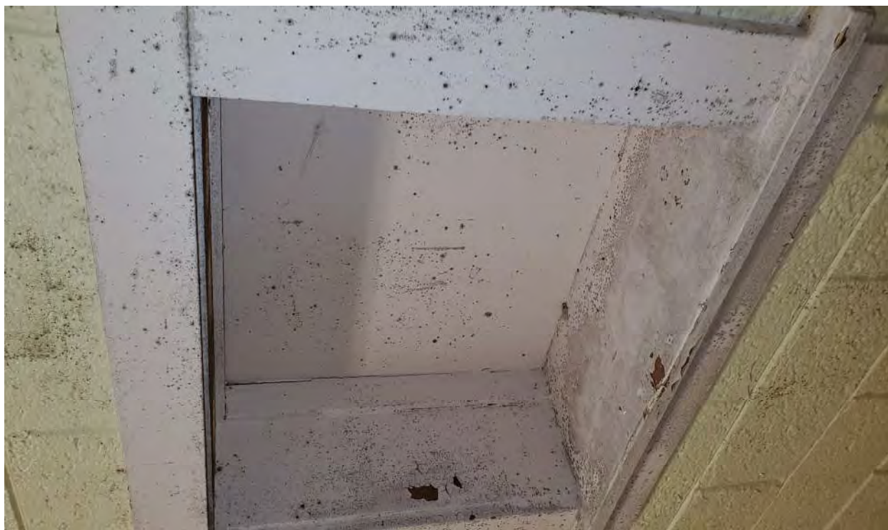
Photograph 11 - Typical Mold Growth on Walls, Door Components, & Other Surfaces Located Throughout the Main Building.
