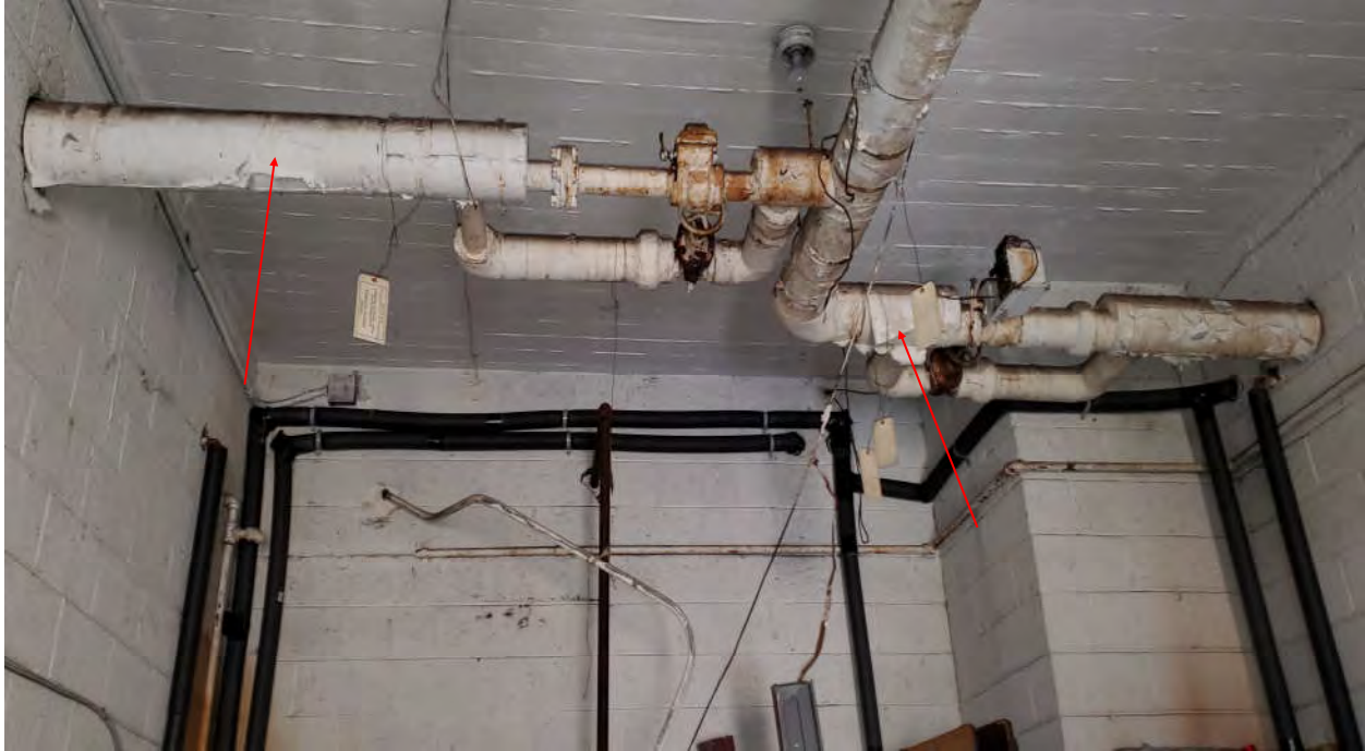
Photograph 5 - Homogeneous Area A-23 - Asbestos-Containing “Air-Cell” Straight Run Pipe Insulation Located Overhead in the Mechanical Room. (10 LF)
