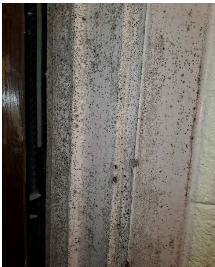
Photograph 10 - Typical Mold Growth on Walls, Door Components, & Other Surfaces Located Throughout the Main Building.
