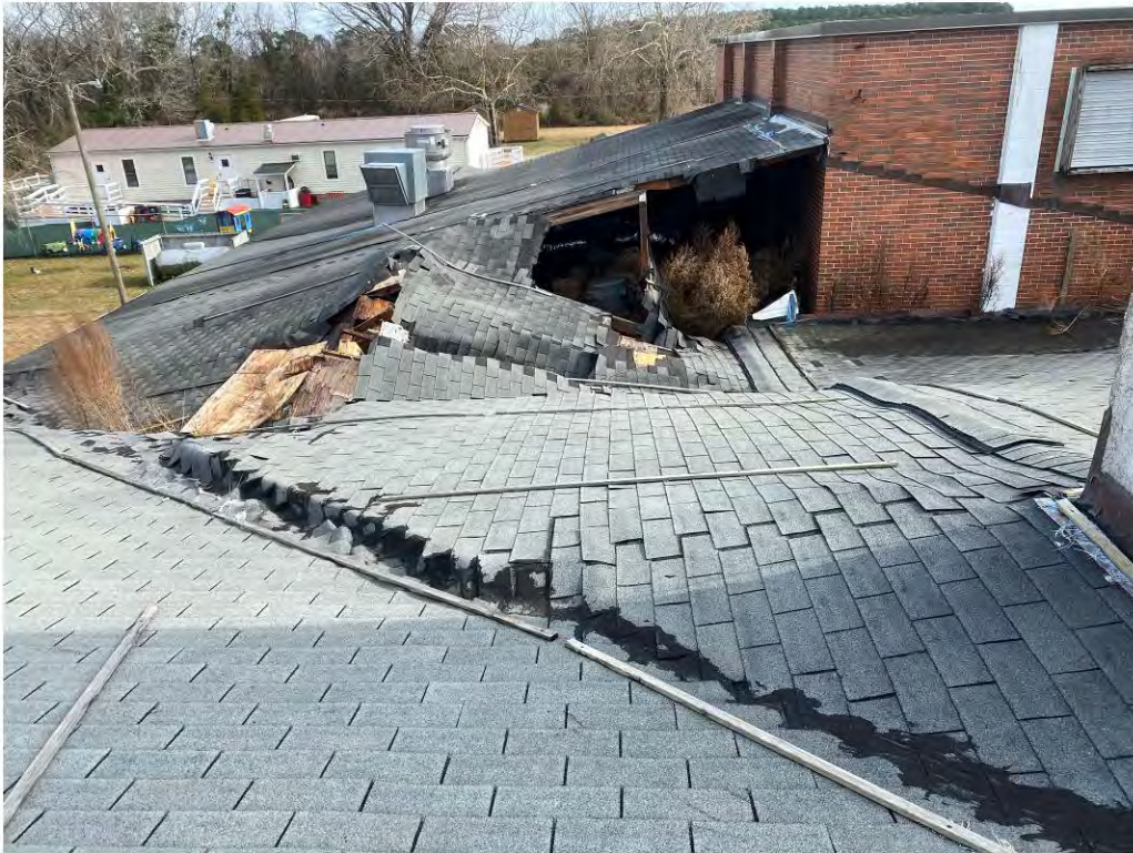
Photograph 11 – Collapsed Roof Area at Right End of Classroom Building
