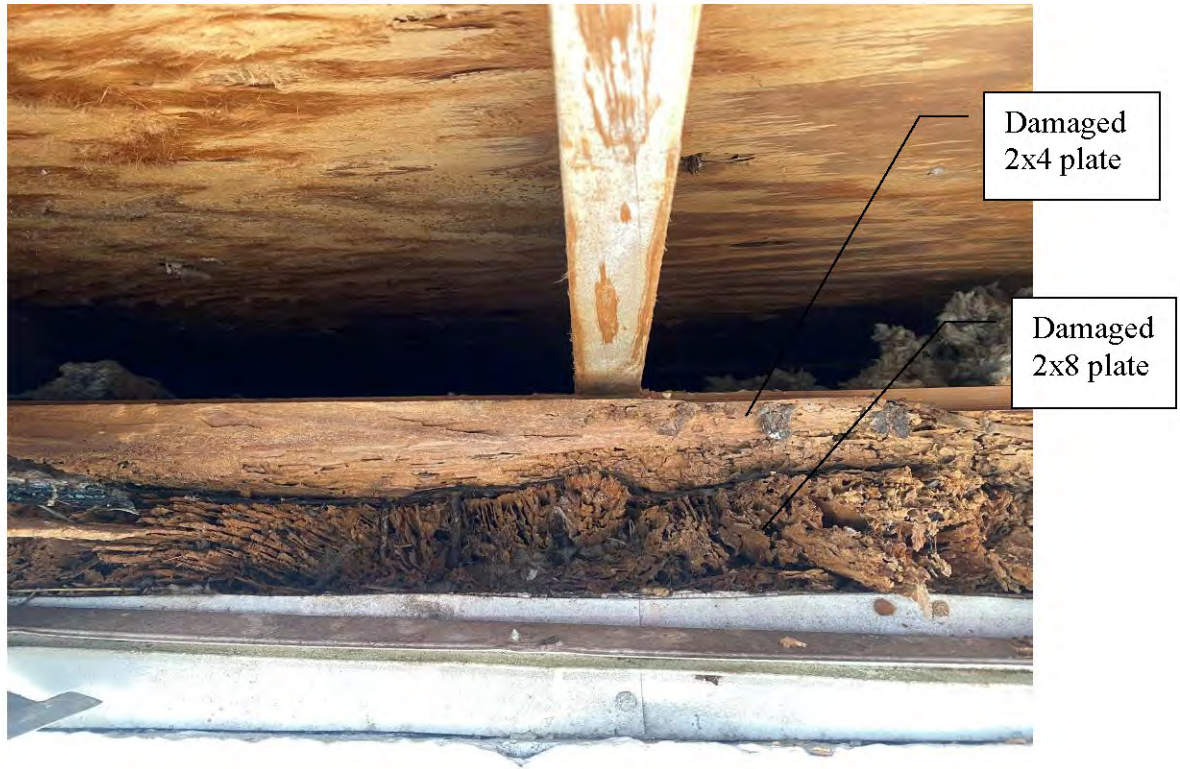
Photograph 9 – Damaged Wood Plating Under Roof Trusses – Classroom Building
