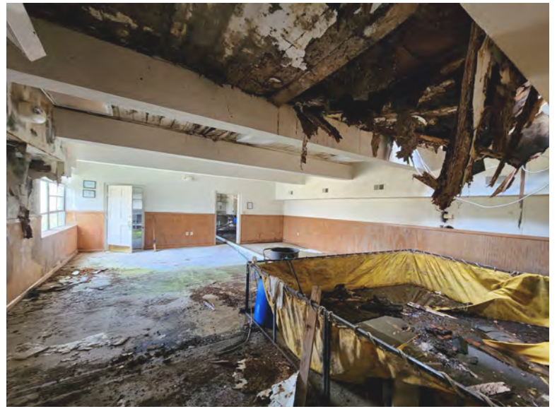
Water damage to dining area. Daylight visible through hole.
