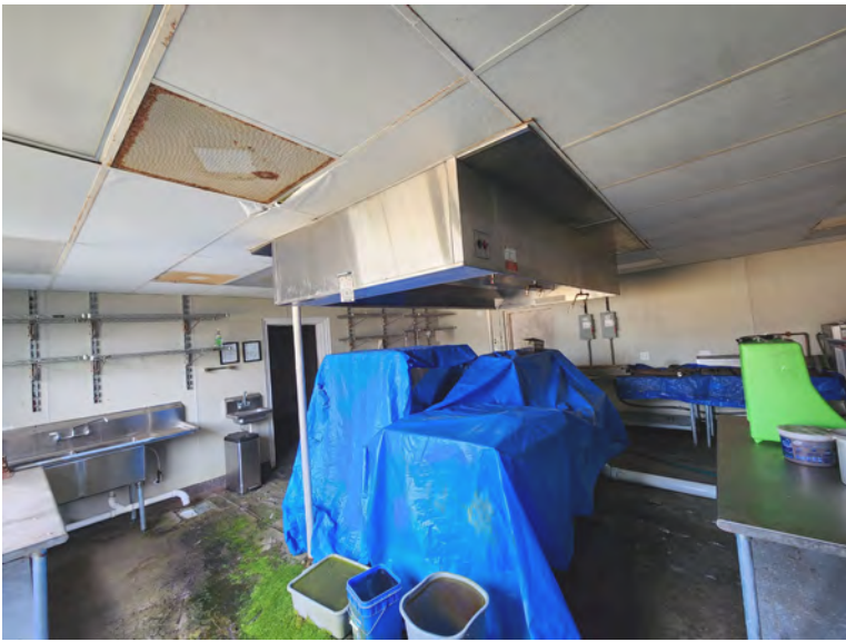
Water damage to commercial kitchen.
