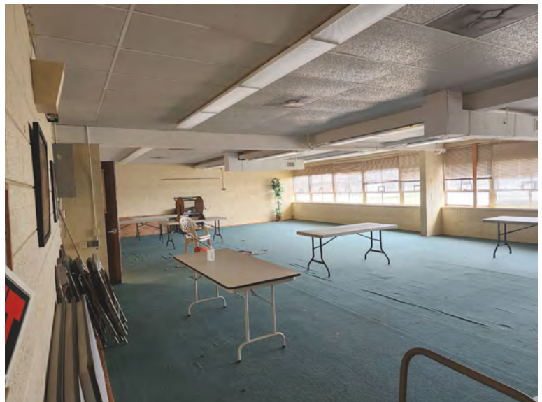
Classroom with evidence of moisture throughout (wrinkled carpet, smell, visible mold, etc.)
