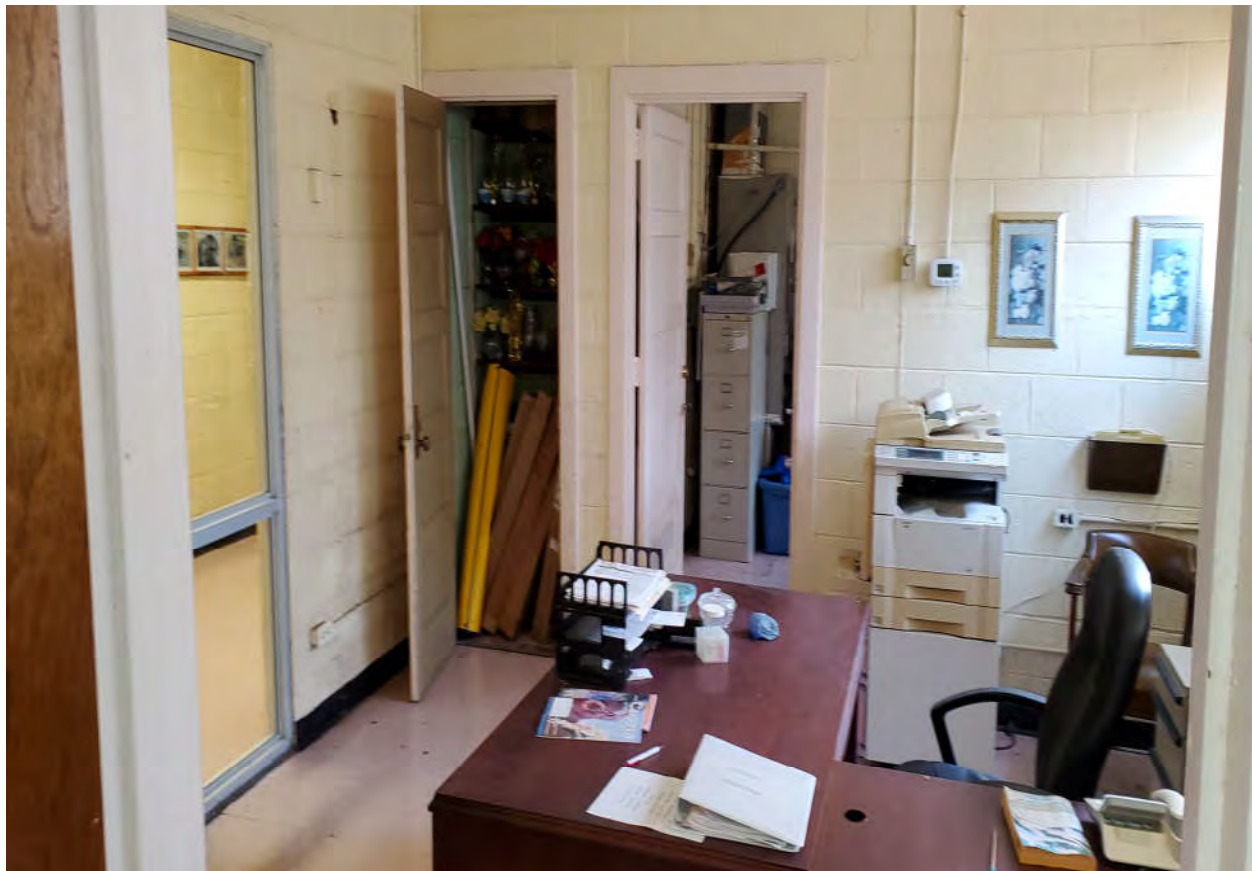
Photograph 8 - Typical Lead-Based Paint on CMU Walls in This One Room Only in Office Area in Main Building.
