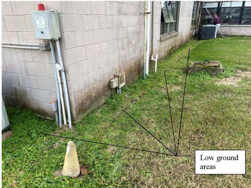
Photograph 13 – Low Ground Areas at Left Side of Gym Connector
