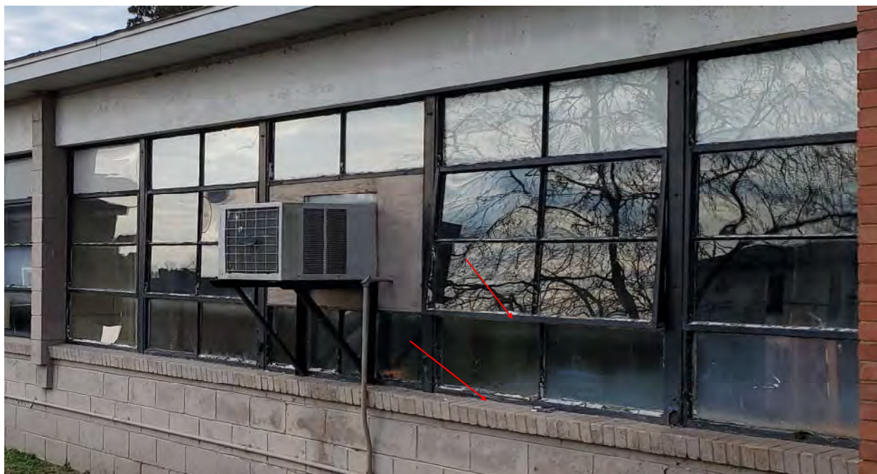
Photograph 1 - Homogeneous Areas A-01 & A-22—Typical Asbestos-Containing Exterior Window Glazing and Window Frame Caulking Located Throughout Main Building Window Units. (57 Window Units)
