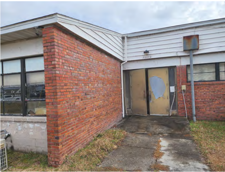
Deteriorating exterior doors.
