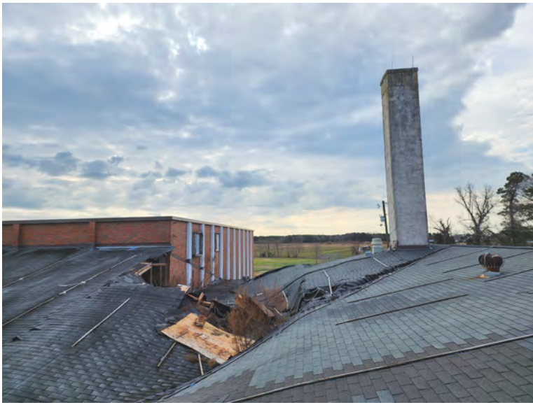
Roof collapse view from the roof.
