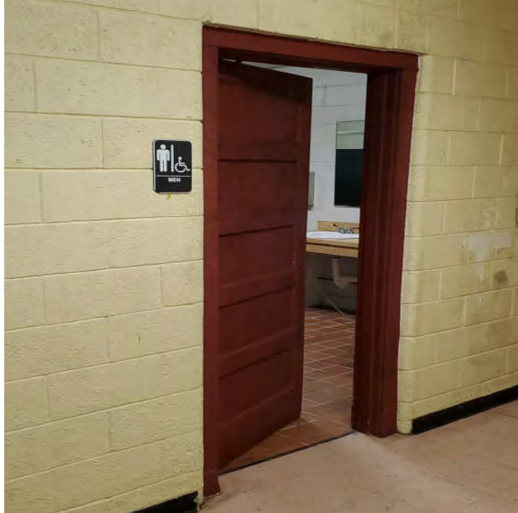
Photograph 7 - Typical Lead-Based Paint on Red Doors and Dooring Casings in Restrooms of Main Building.
