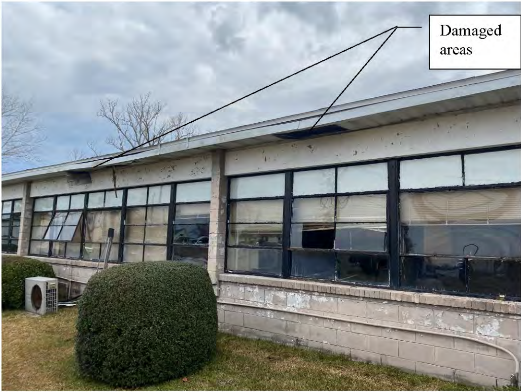
Photograph 8 – Damaged Soffit Areas – Front of Classroom Building
