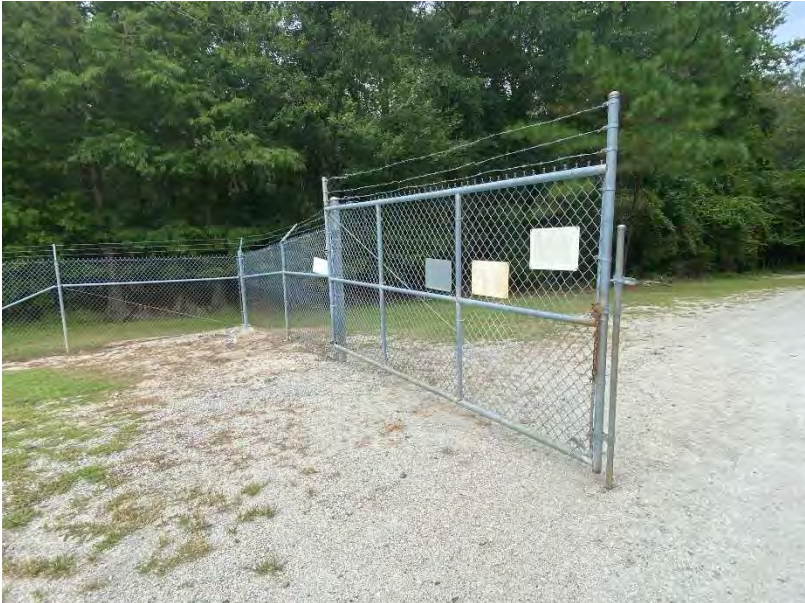
Photo No. 8 Entry Gate System
