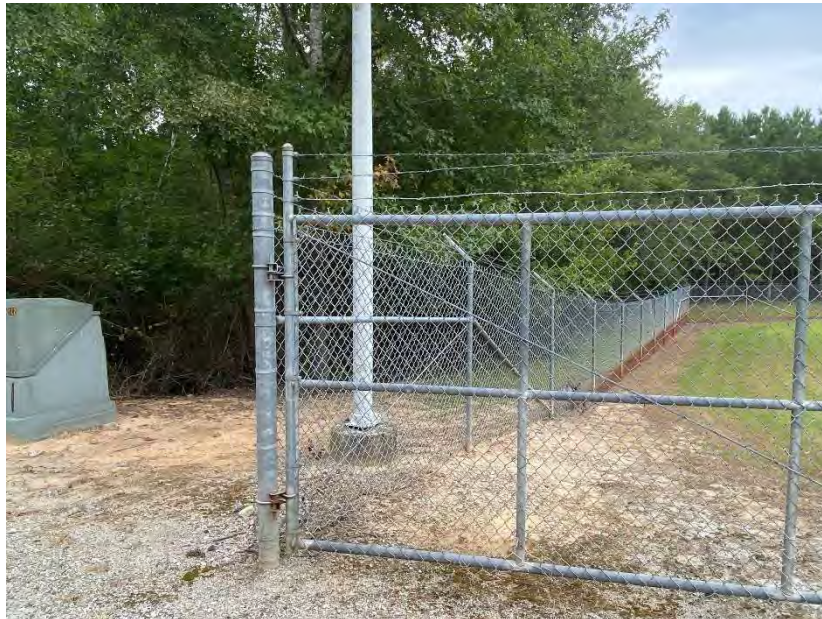
Photo No. 7 Entry Gate System
