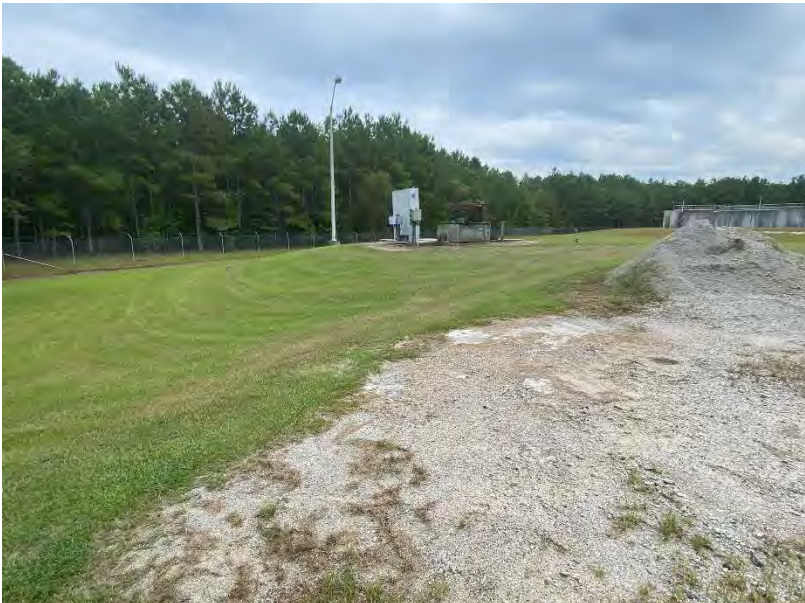
Photo No. 10 Lift Station
