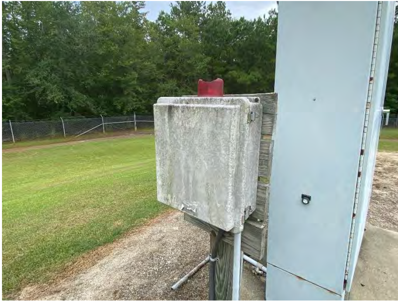
Photo No. 11 Lift Station Control Panel
