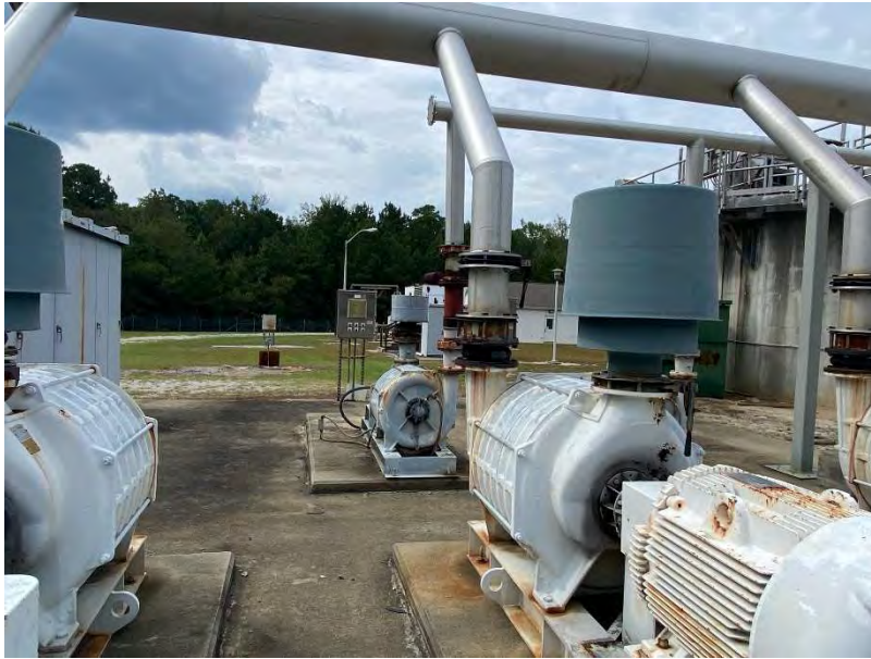
Photo No. 17 Plant Control Equipment
