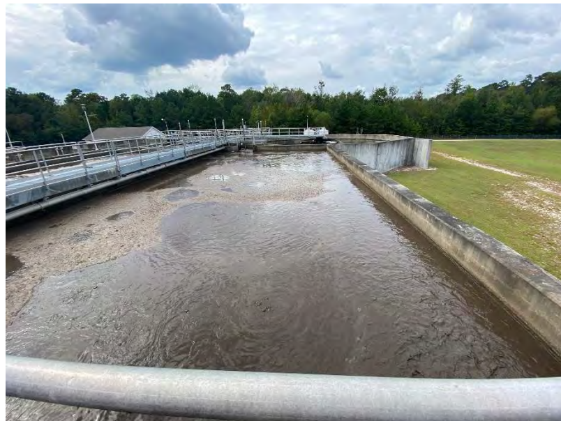
Photo No. 20 Effluent Pond (Height Due to Storm-Damaged Gates)
