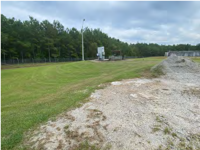
Photo No. 10 Lift Station
