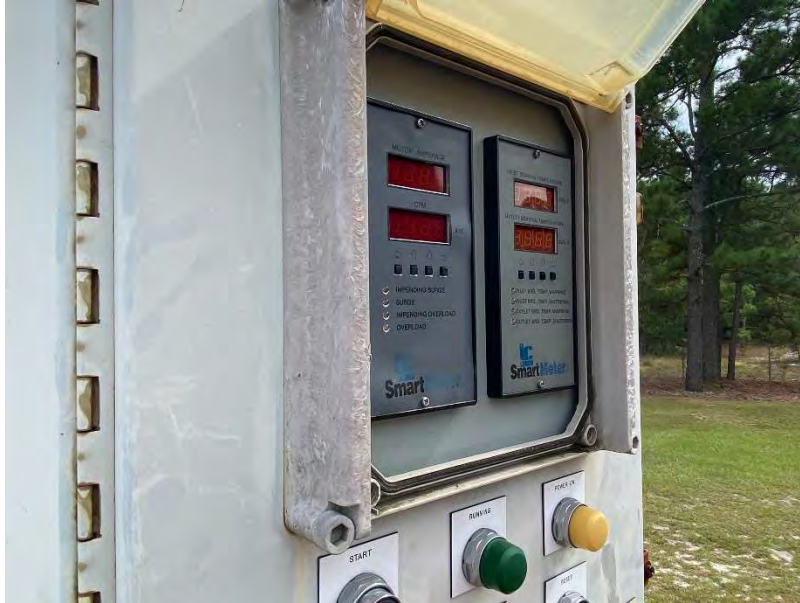
Photo No. 6 1980's Control Unit
