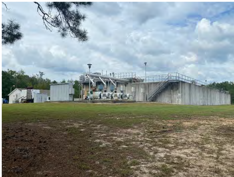
Photo No. 16 Fairmont Wastewater Treatment Plant Facing Northwest
