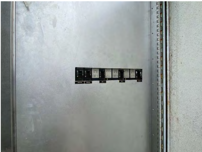
Photo No. 12 Lift Station Electrical Panel
