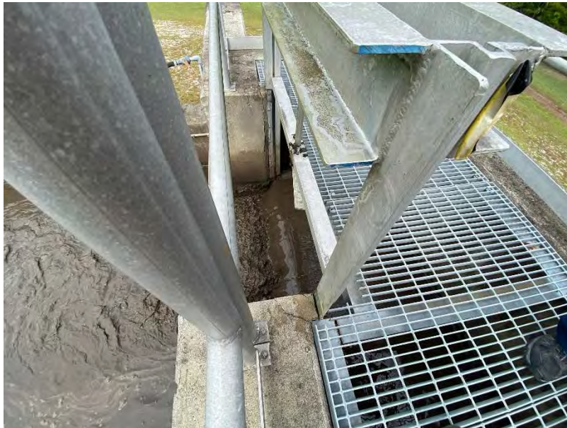
Photo No.18 Broken Effluent Gate
