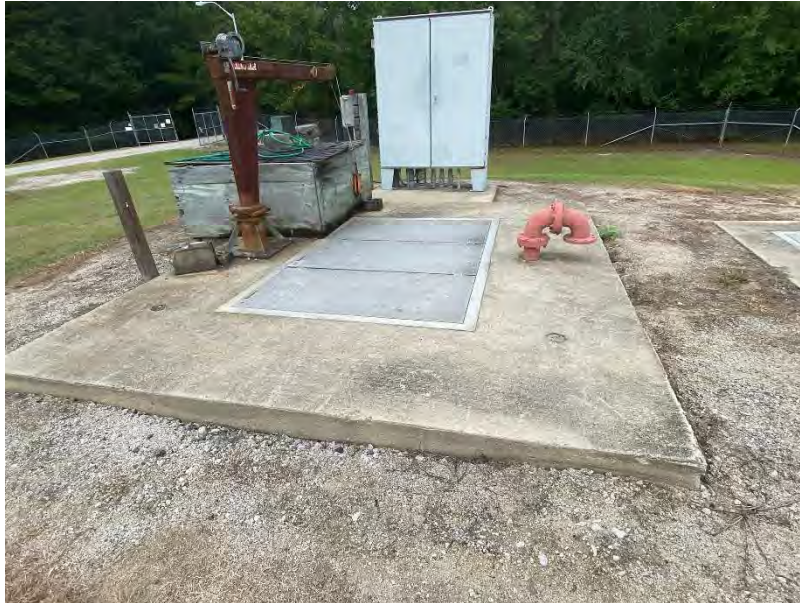
Photo No. 15 Lift Station Equipment
