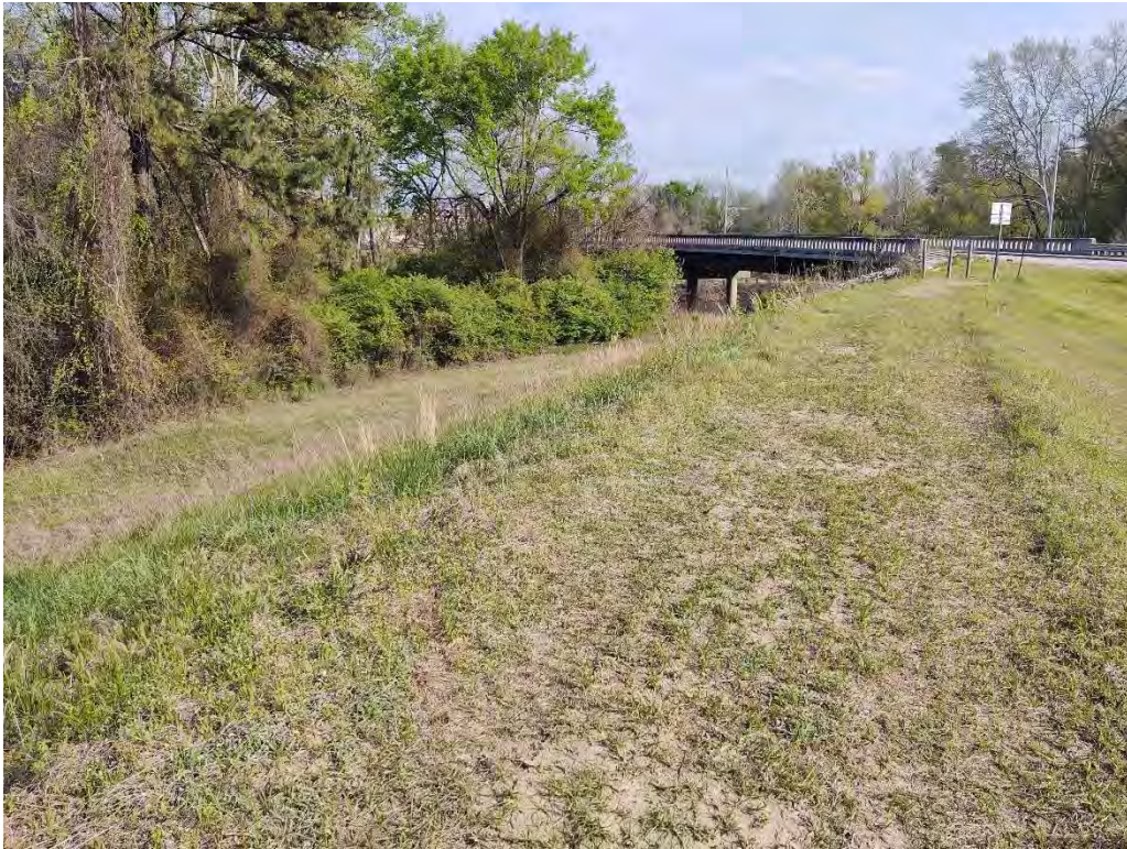
RS 245115 - Top of Levee Looking North Toward NC 33 Bridge over Tar River
