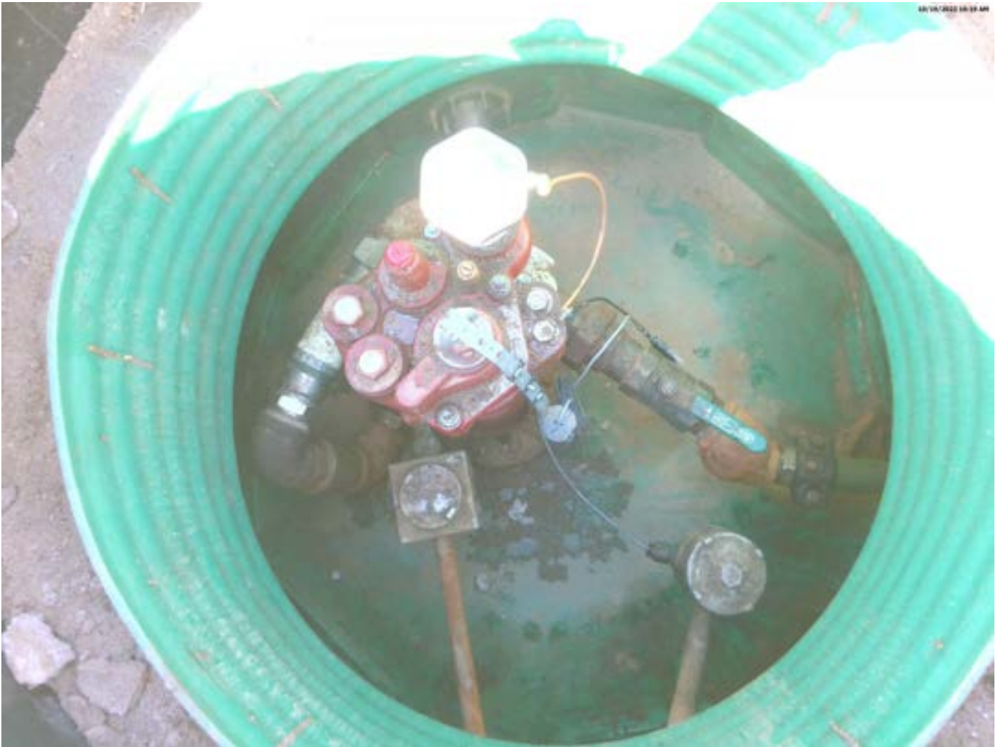
PICDIAG DIESEL STP SUMP
