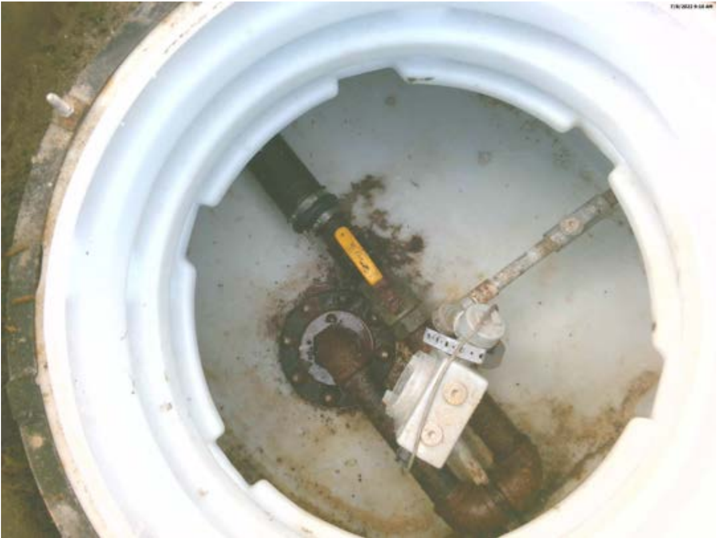
PICDIAG DIESEL TANK TOP SUMP
