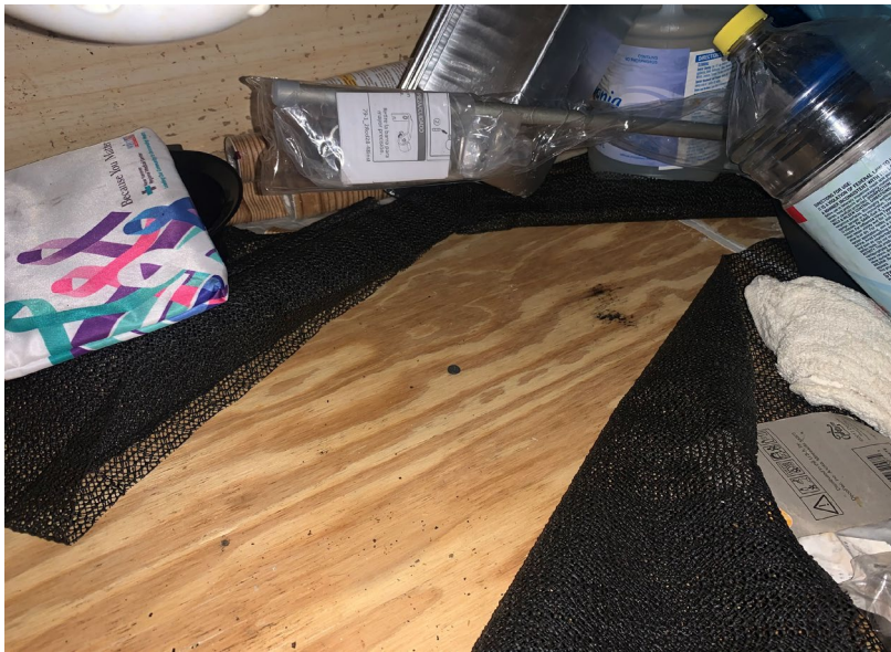
Suspect visible mold growth in the kitchen cabinet underneath sink.
