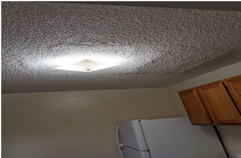
Apparent water damage to the kitchen ceiling
