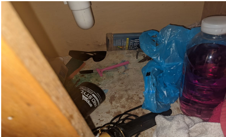
Apparent water damage and buckling in the bathroom cabinet
