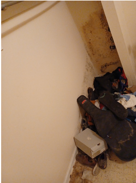
Suspect visible mold growth on the rear left bedroom closet walls
