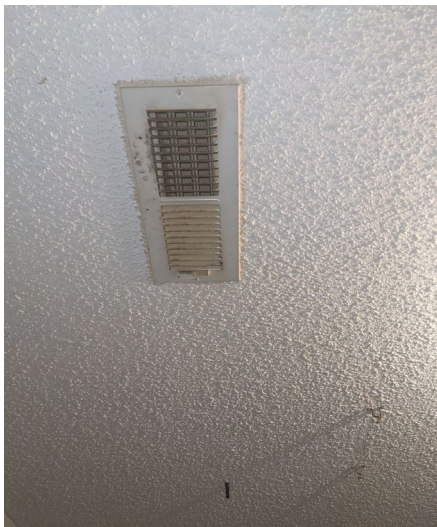
Suspect visible mold growth on the HVAC supply vent in the living room
