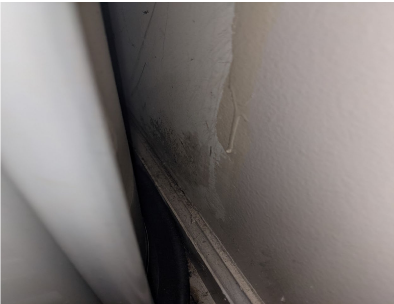
Suspect visible mold growth on the rear left bedroom closet right wall (adjacent to the water heater)
