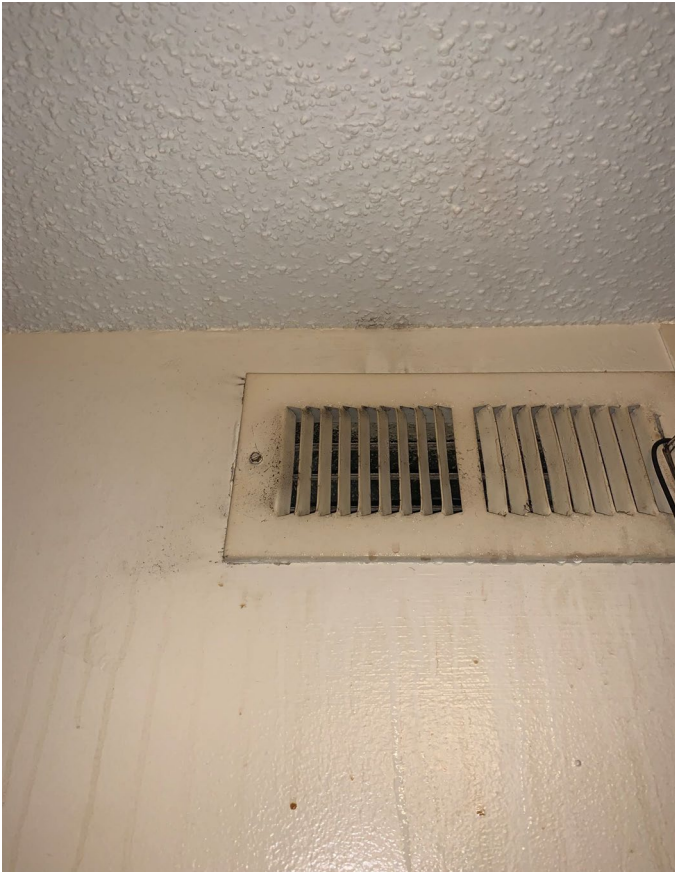
Suspect visible mold growth/dust on the HVAC supply vent in the rear right bedroom
