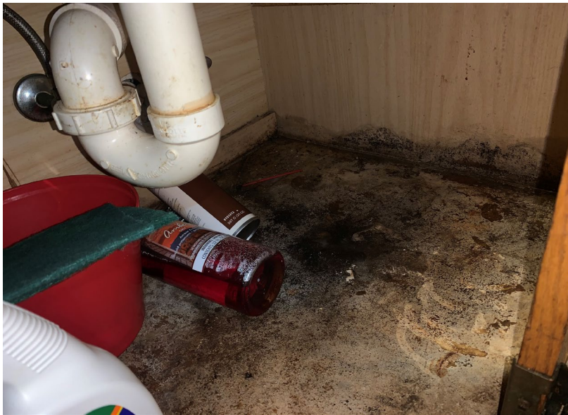
Apparent water damage and suspect visible mold growth in kitchen cabinet underneath sink
