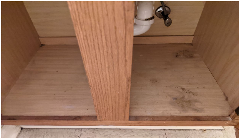
Apparent water damage to the bathroom cabinet
