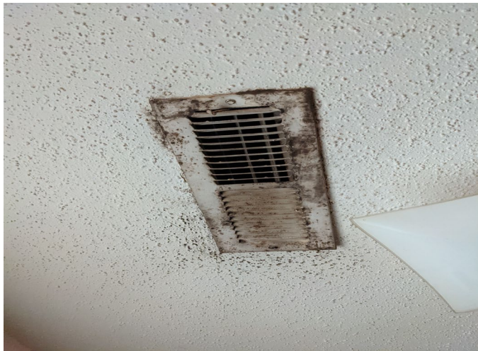
Suspect visible mold growth on the kitchen HVAC supply vent
