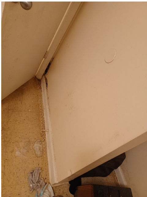
Suspect visible mold growth on the rear left bedroom front and front right walls
