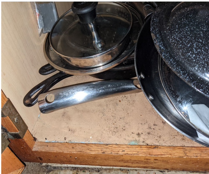
Suspect visible mold growth on the rear cabinets in the kitchen
