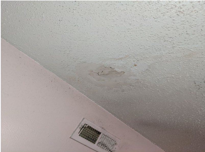
Apparent water damage to the ceiling/hole in the rear right bedroom
