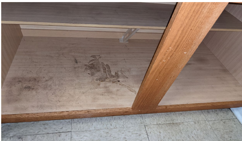
Apparent water damage in the kitchen floor mounted cabinet on the rear wall (left side)
