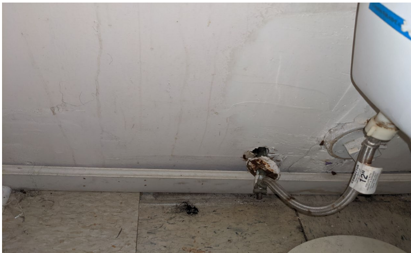
Apparent water damage to the bathroom front wall baseboard
