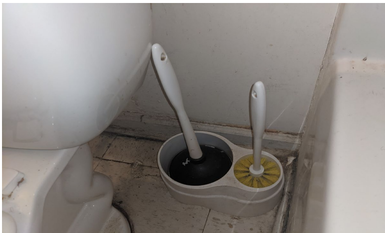
Apparent water damage on the bathroom front wall baseboard
