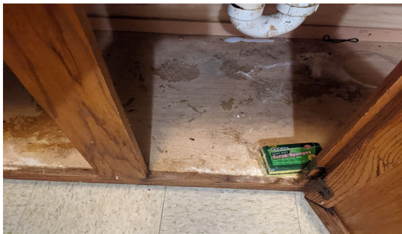
Apparent water damage in the kitchen cabinet on the front wall
