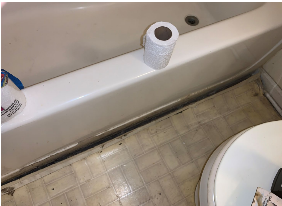
Apparent water damage on the floor in the bathroom near the bathtub
