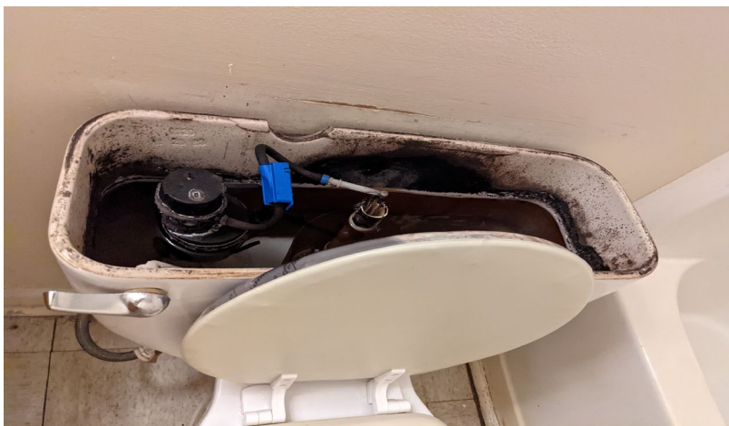
Suspect visible mold growth in the bathroom toilet tank
