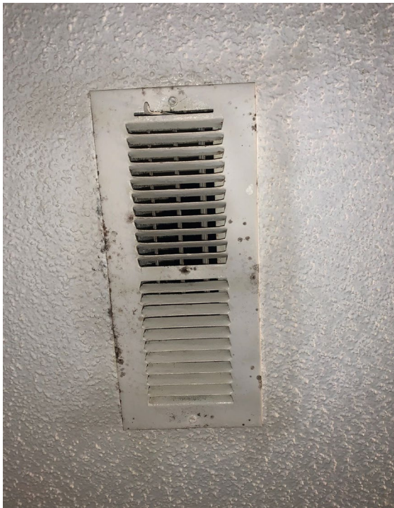
Suspect visible mold growth on the HVAC supply vent in the rear left bedroom
