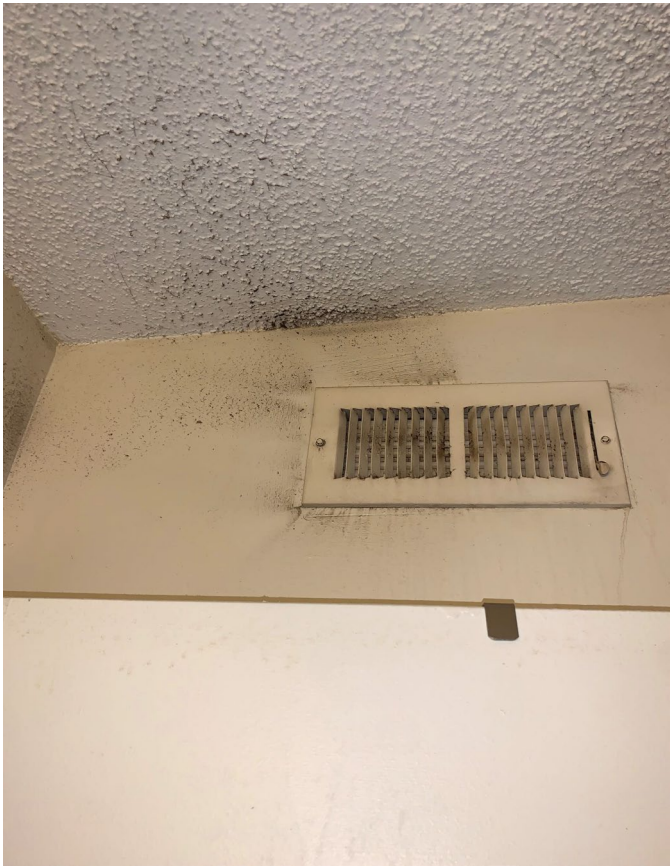
Suspect visible mold growth/dust on and around the HVAC supply vent in the bathroom
