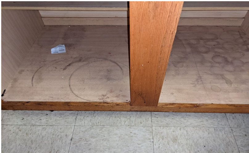
Apparent water damage in the kitchen floor mounted cabinet on the rear wall (right side)
