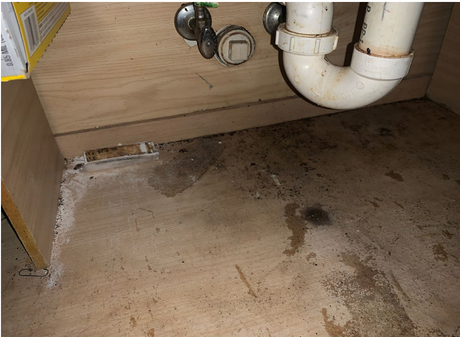
Apparent water damage/suspect visible mold growth in kitchen cabinet underneath sink
