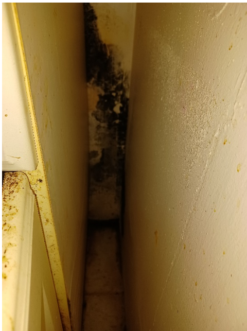
Suspect visible mold growth on the bathroom front wall
