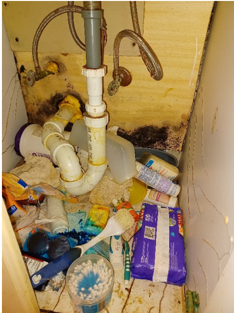
Suspect visible mold growth in the bathroom cabinet
