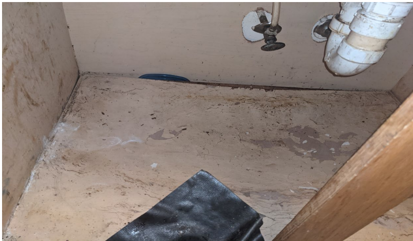
Apparent water damage and Suspect visible mold growth in the kitchen front floor mounted cabinet
