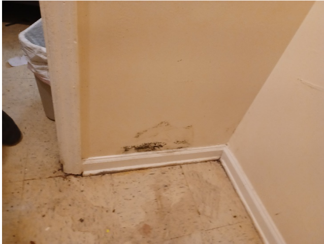
Suspect visible mold growth on the rear right bedroom rear left wall
