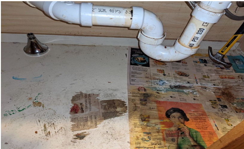
Apparent water damage within the kitchen sink cabinet
