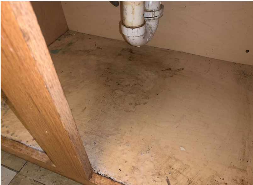
Apparent water damage in the bathroom cabinet underneath the sink
