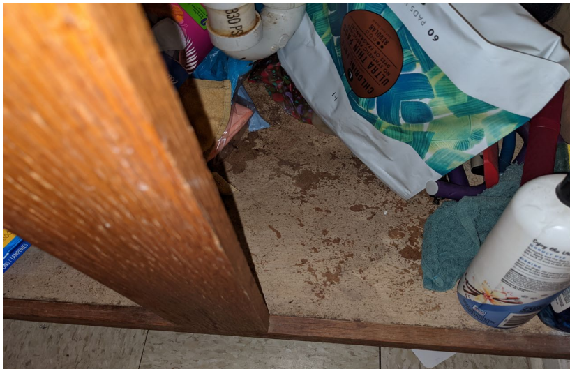
Apparent water damage within the bathroom cabinet on the front wall
