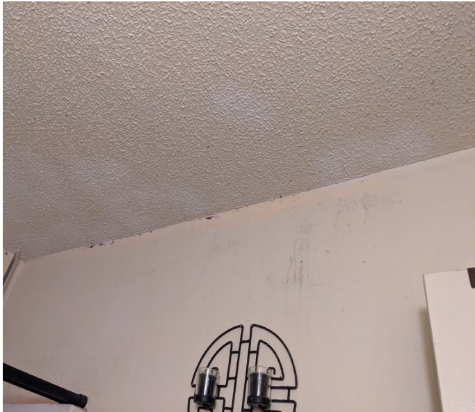
Suspect visible mold growth on the rear wall in the bathroom
