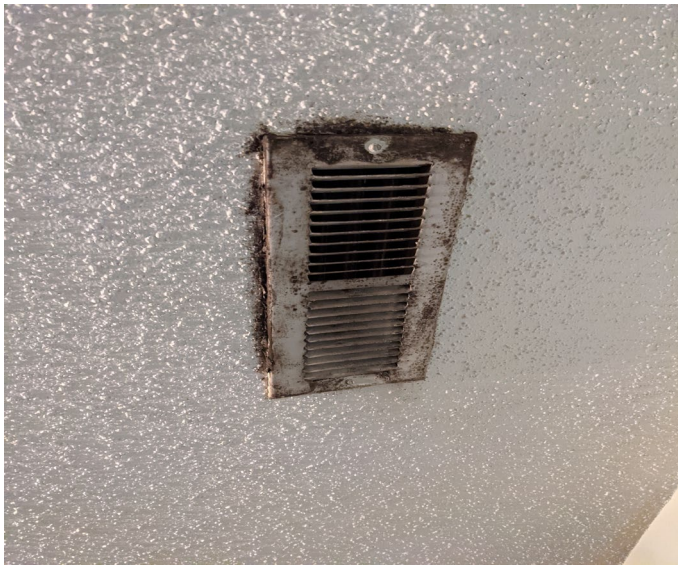
Suspect visible mold growth on the living room HVAC supply vent
