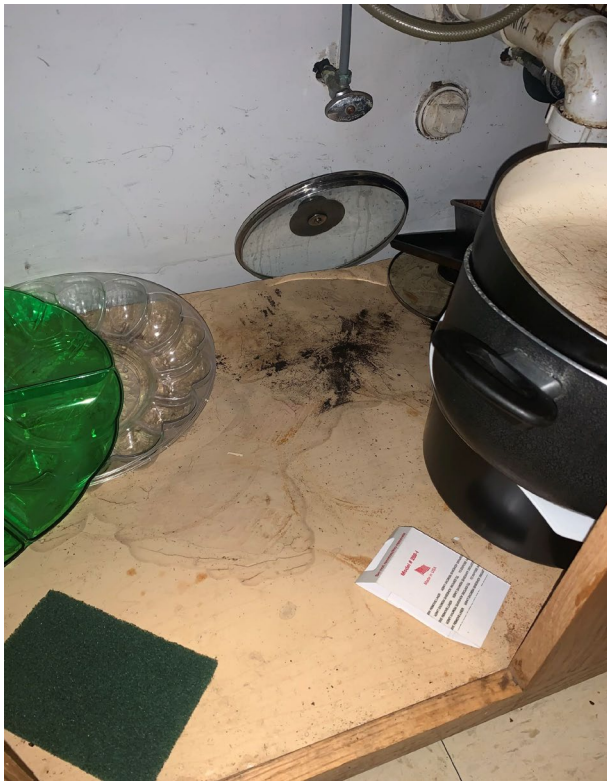
Apparent water damage/suspect visible mold growth in the kitchen cabinet underneath the sink
