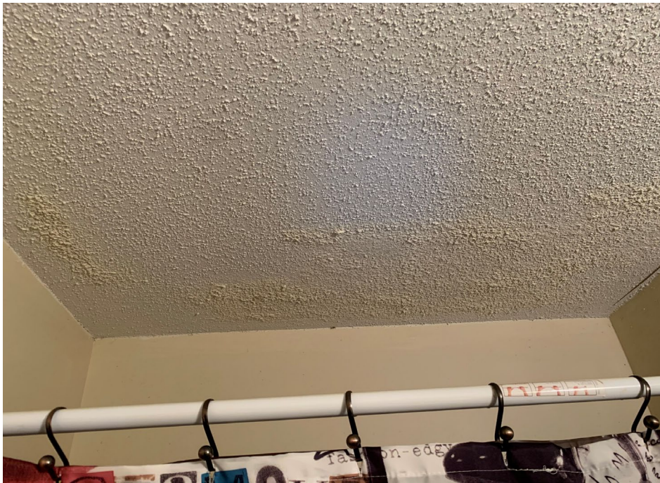
Apparent water damage/discoloration on the bathroom ceiling
