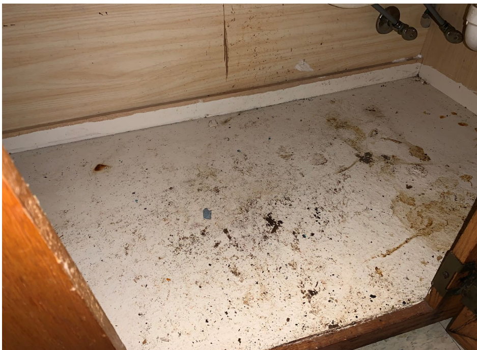
Apparent minor water damage/staining in the cabinet underneath the kitchen sink
