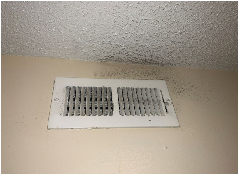
Dust/suspect visible mold growth on and around the HVAC supply vent in rear right bedroom
