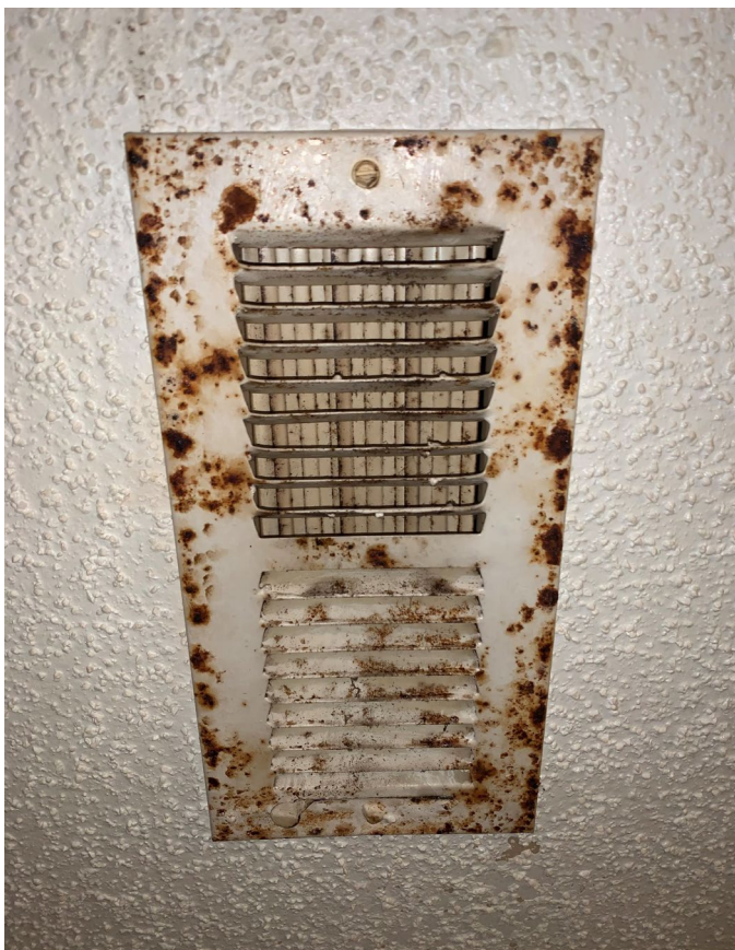
Suspect visible mold growth and rust on the HVAC supply vent in the bathroom
