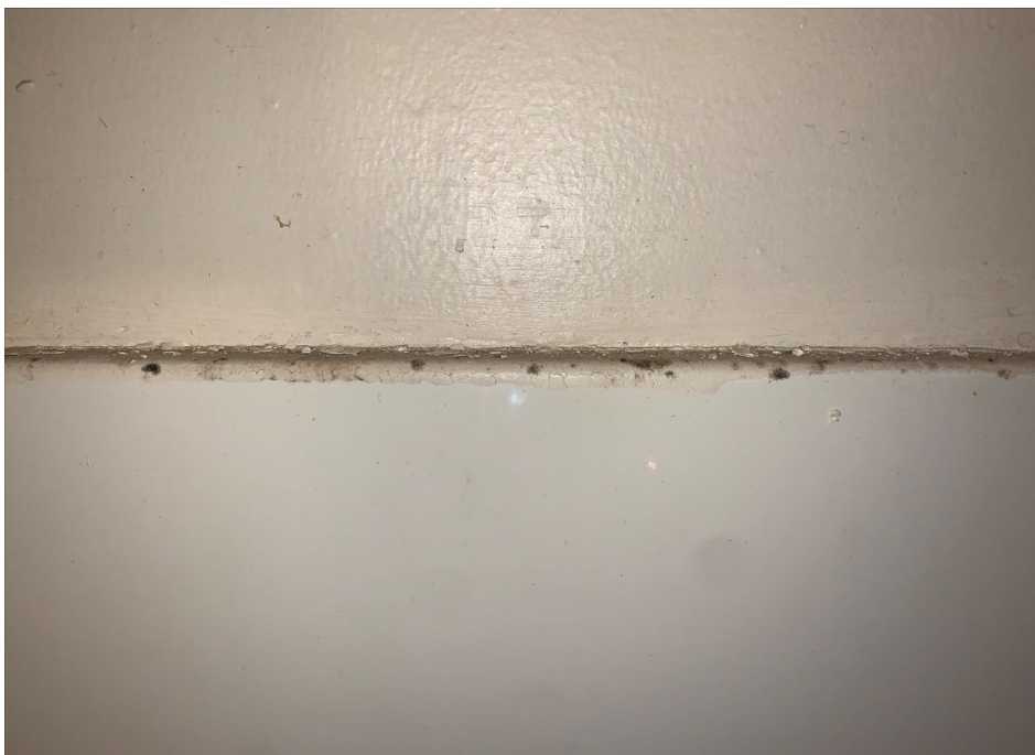
Suspect visible mold growth on the bathroom bathtub
