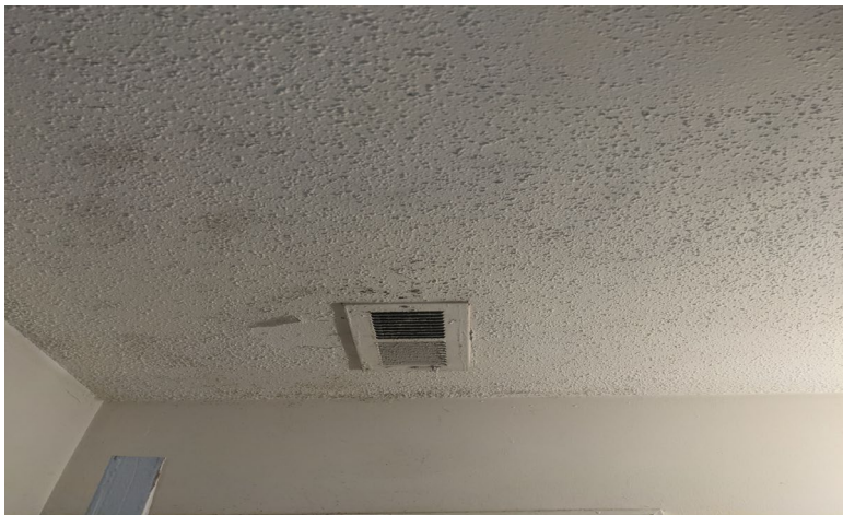
Suspect visible mold growth on the walls and the HVAC supply vent in the bathroom
