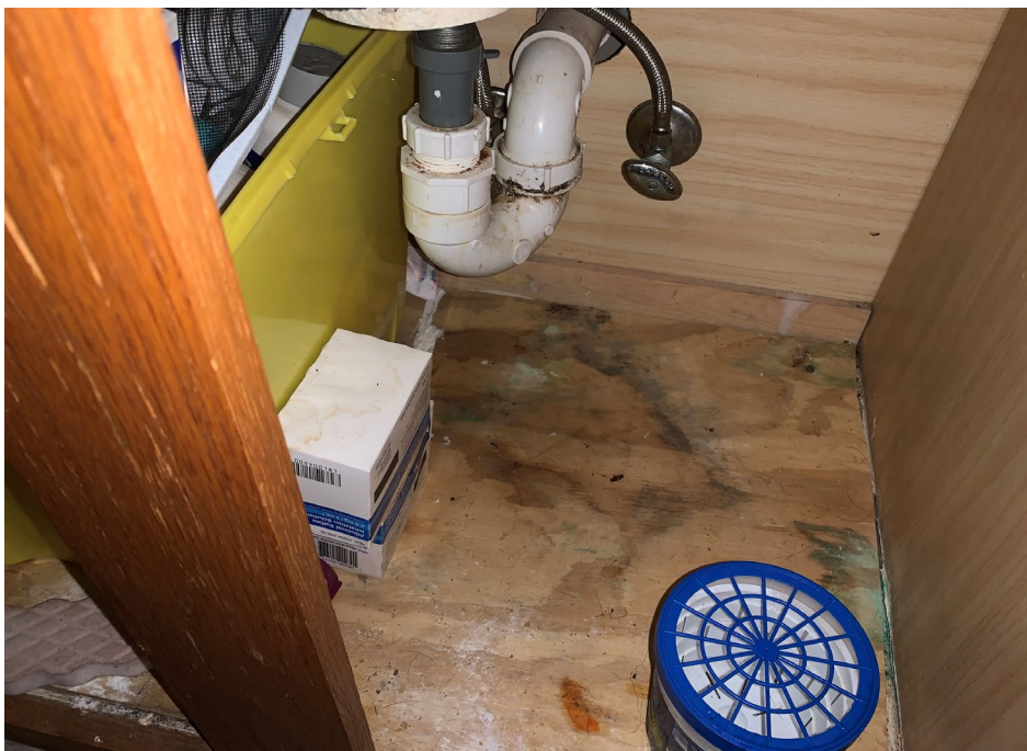
Apparent water damage and suspect visible mold growth in the bathroom cabinet under the sink
