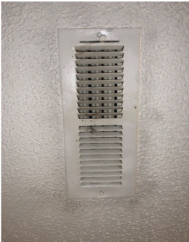
Suspect visible mold growth on the HVAC supply vent in the rear right bedroom
