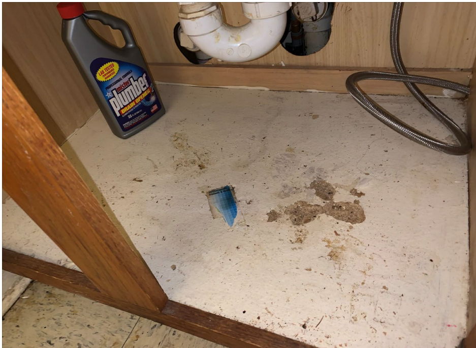
Apparent minor water damage/staining in the cabinet underneath the bathroom sink
