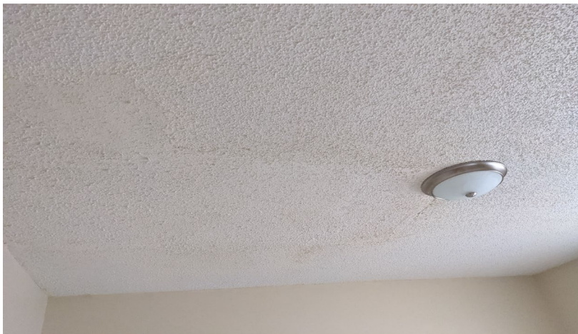
Apparent water damage to the ceiling in the front left bedroom
