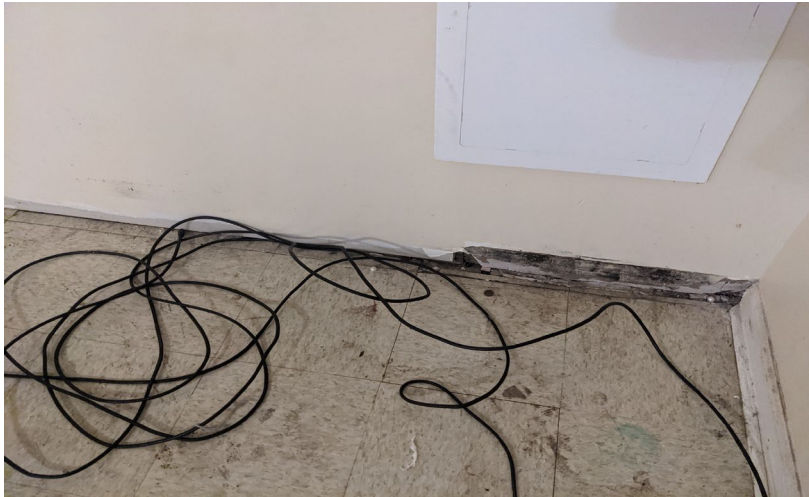
Suspect visible mold growth on the living room rear wall
