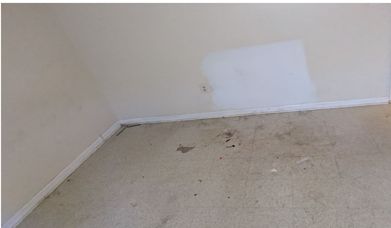
Apparent water damage to the front right bedroom rear and right baseboards
