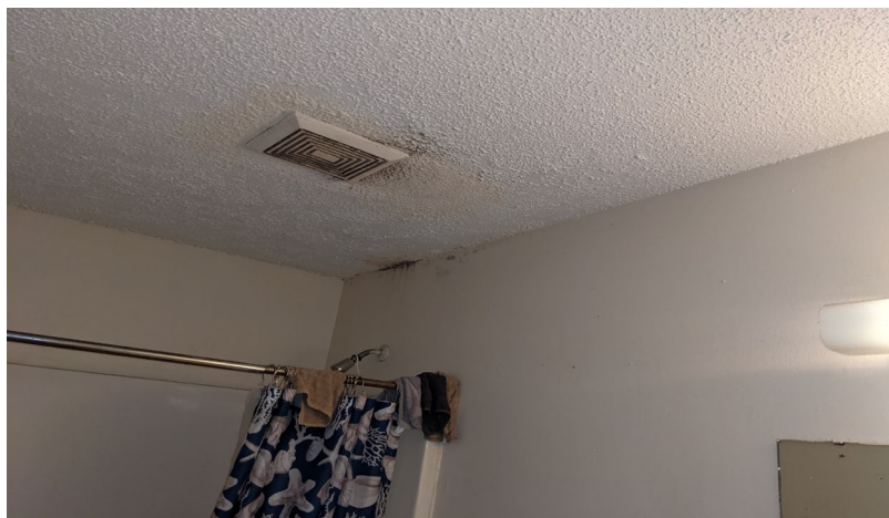
Apparent water damage and suspect visible mold growth on the bathroom ceiling and front wall
