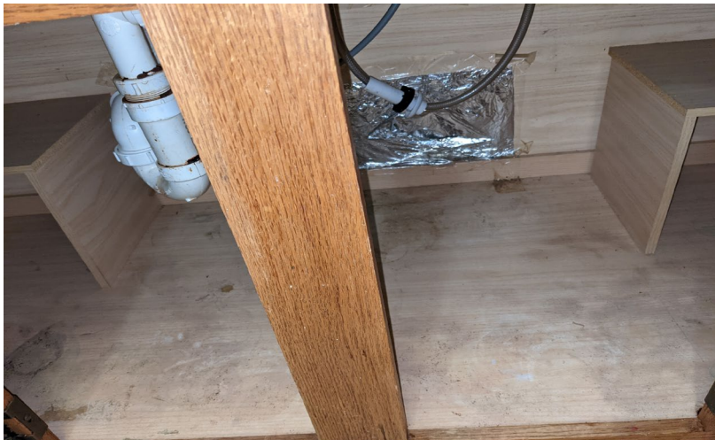
Apparent water damage in the kitchen floor mounted cabinet on the front wall
