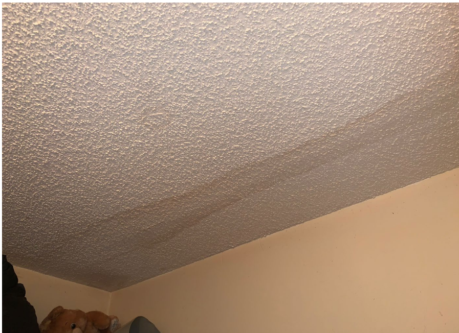
Apparent water damage on the ceiling in the closet of the rear left bedroom
