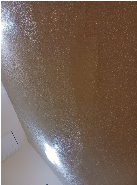
Apparent water damage on the living room ceiling
