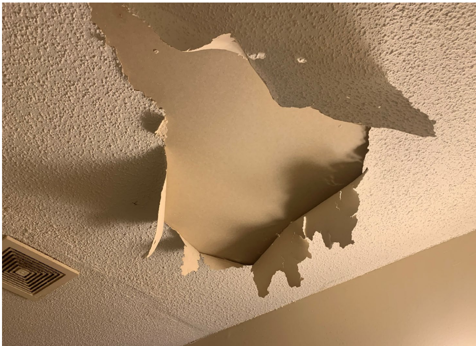
Paint peeling from the ceiling in the bathroom
