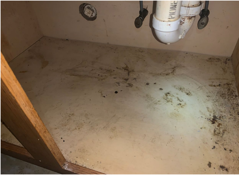
Apparent water damage in the kitchen cabinet underneath the sink
