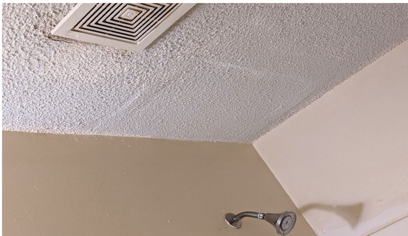
Apparent water damage to the bathroom ceiling
