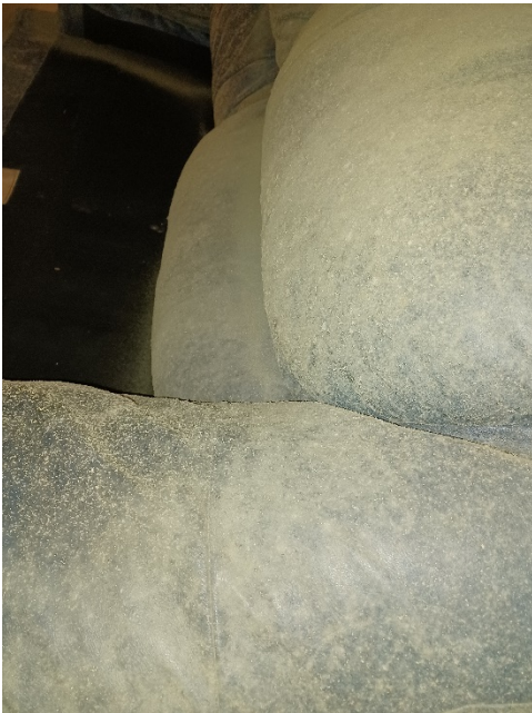
Suspect visible mold growth on furniture in the living room
