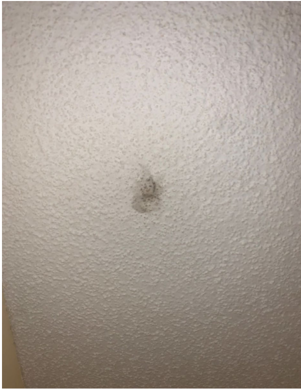
Apparent water damage to the popcorn ceiling in the rear right bedroom
