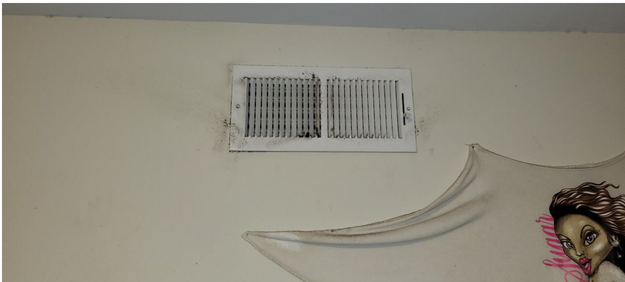
Dust/suspect visible mold growth on HVAC supply vents in various locations throughout. Note: Photo taken in the 2 nd floor front right bedroom
