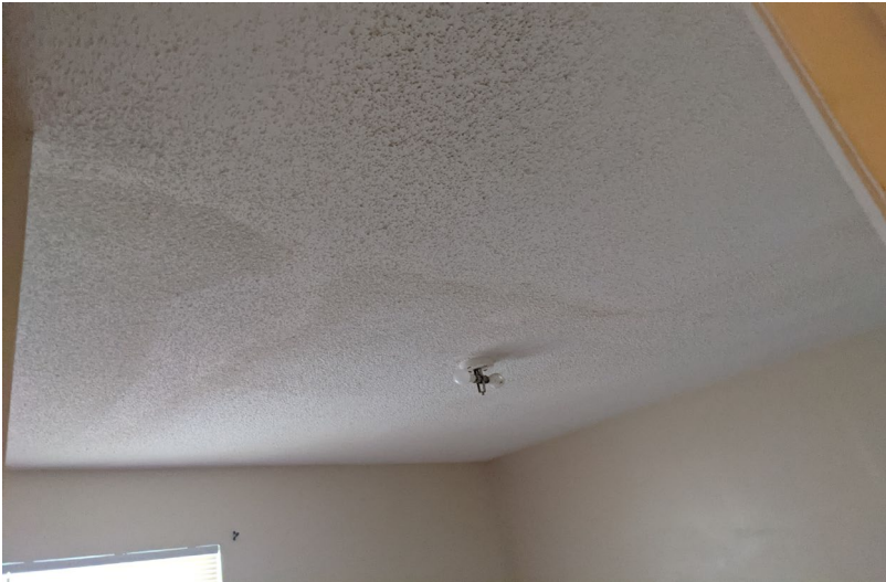
Apparent water damage/irregularity to the front right bedroom ceiling
