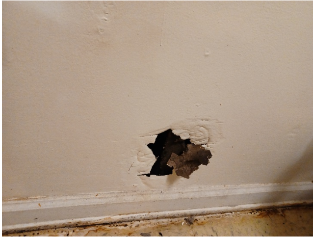
Hole and suspect visible mold growth in the living room rear wall
