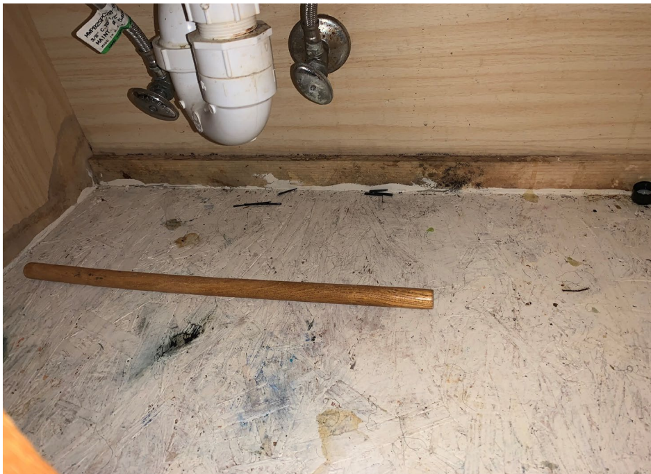
Apparent water damage/suspect visible mold growth in the bathroom cabinet underneath sink
