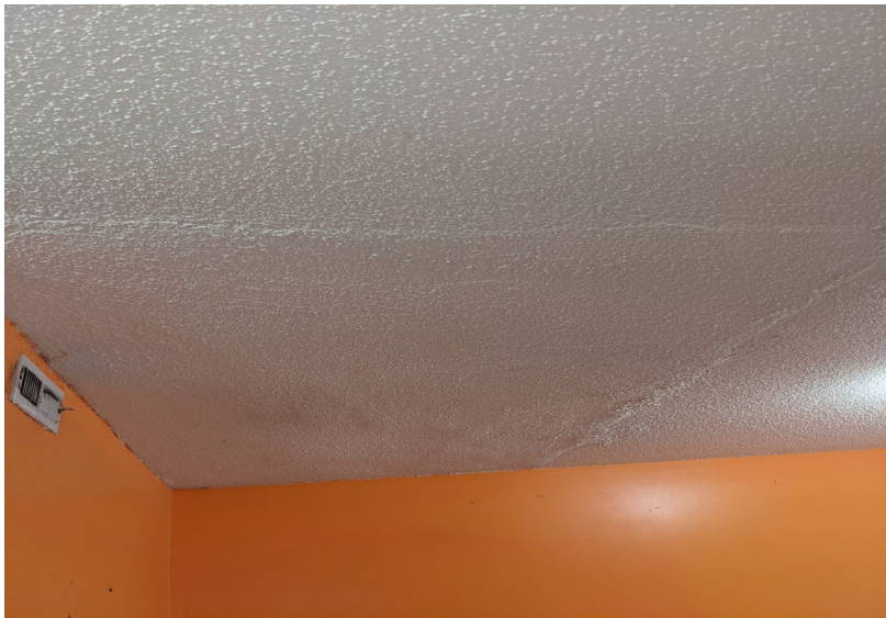
Apparent water damage to the living room ceiling
