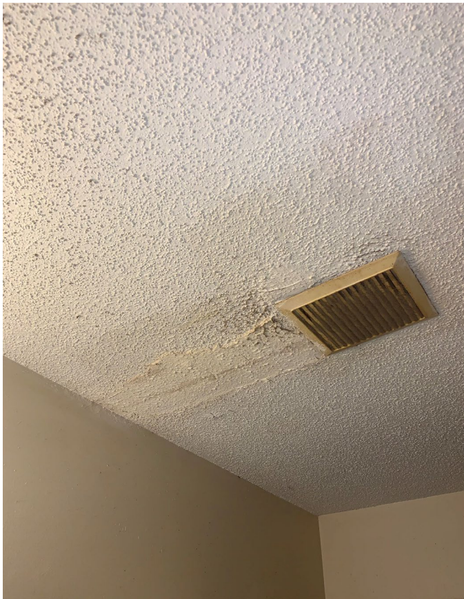
Apparent water damage on the ceiling in the rear left bedroom
