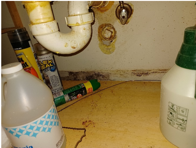
Suspect visible mold growth in the kitchen floor mounted cabinet on the front wall
