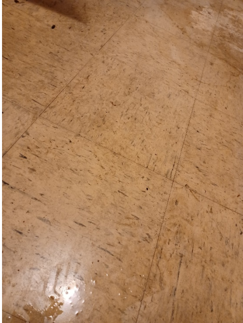
Standing water on the kitchen floor
