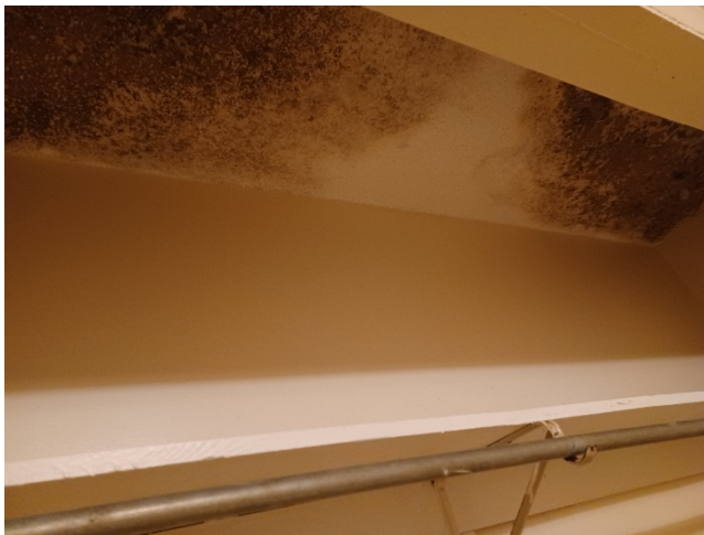
Suspect visible mold growth on the rear left bedroom closet ceiling
