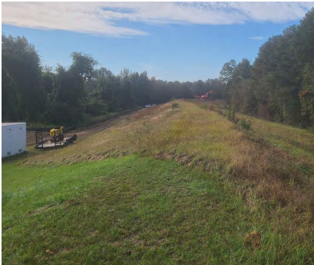
RS 245115 - Top of Levee Looking South Toward R.R. Crossing over Tar River
