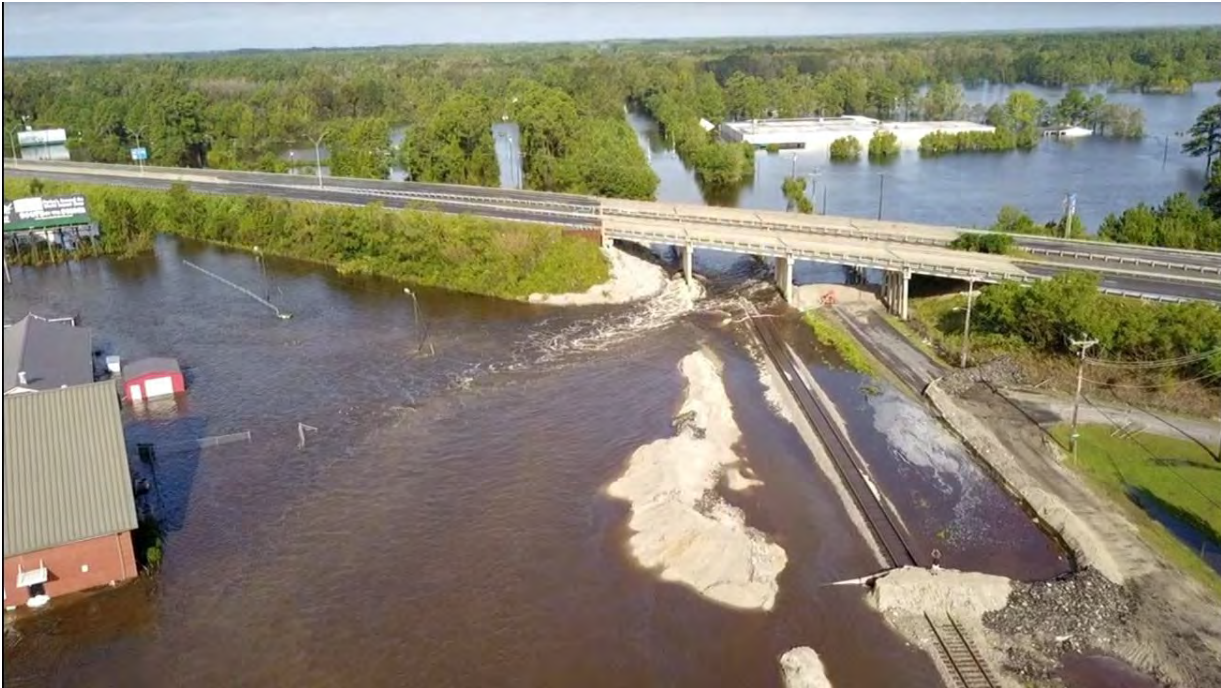
Figure 2-3. Flooding under I-95 at VFW Road and CSX railroad in Lumberton, NC from Hurricane Florence (Source: City of Lumberton).
